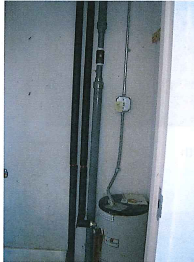
Passive vent room vent pipe
