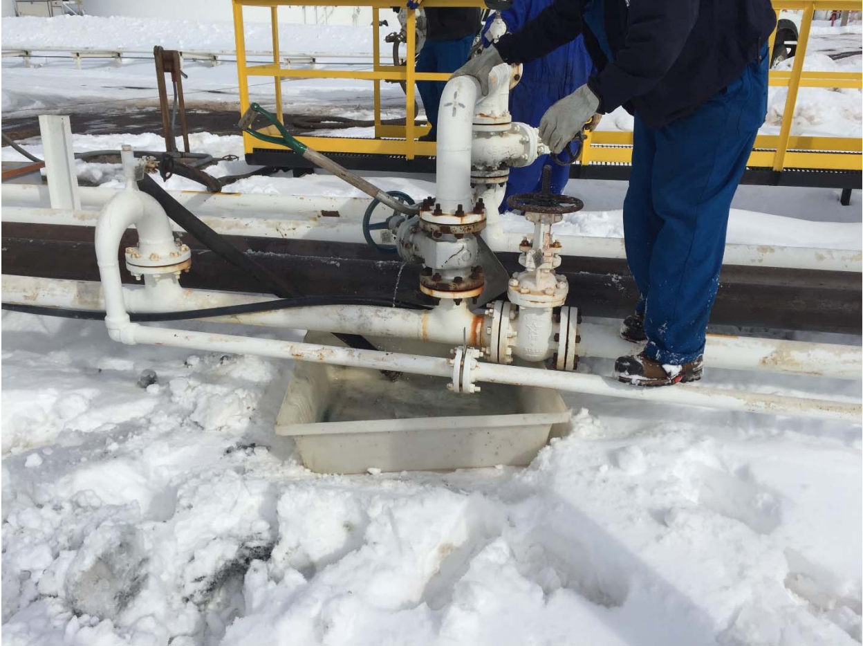
Photo 1: Looking east at the leaking valve. Note the stream of naphtha coming from the gasket on the body of the valve. A plastic container was installed to catch the material and a vacuum truck hose can be seen recovering the material from the container.
