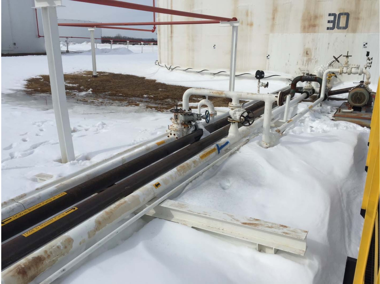
Photo 2: Looking northwest at the release site. The leaking valve is pictured in the center of the image.
