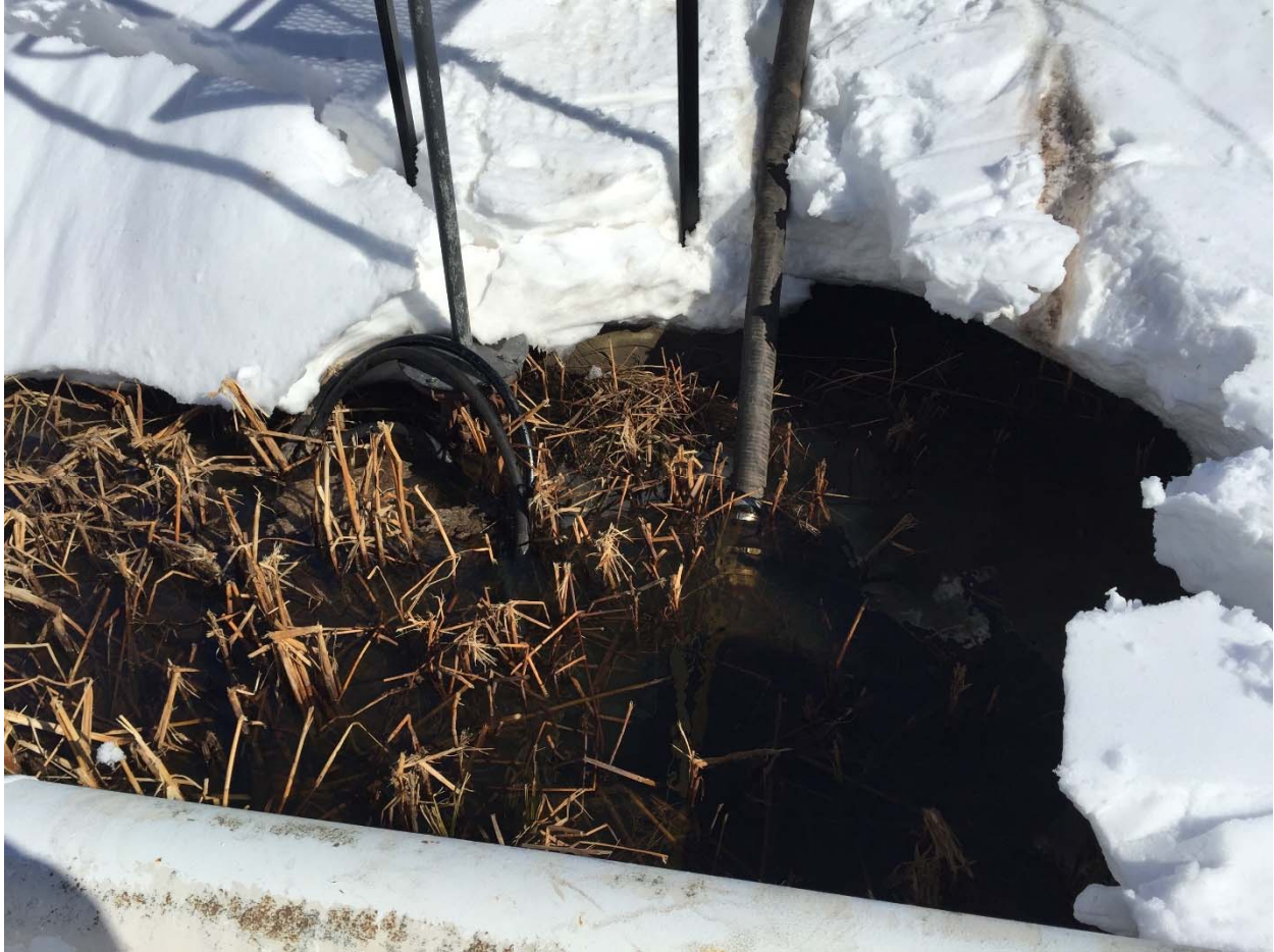
Photo 5: Looking east at the tank dike drain valve pooling location. Steam coils were placed to melt the snow and ice to allow vacuum trucks to collect the recoverable product and contaminated water.
