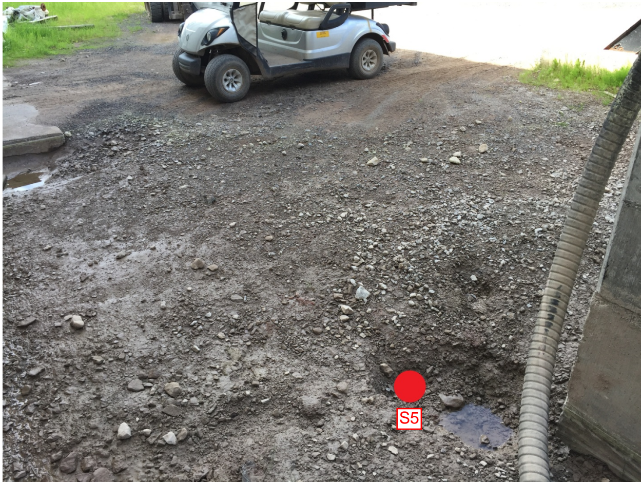
Photo 10: Looking northwest at the excavation and sample location of S5 (red dot).
