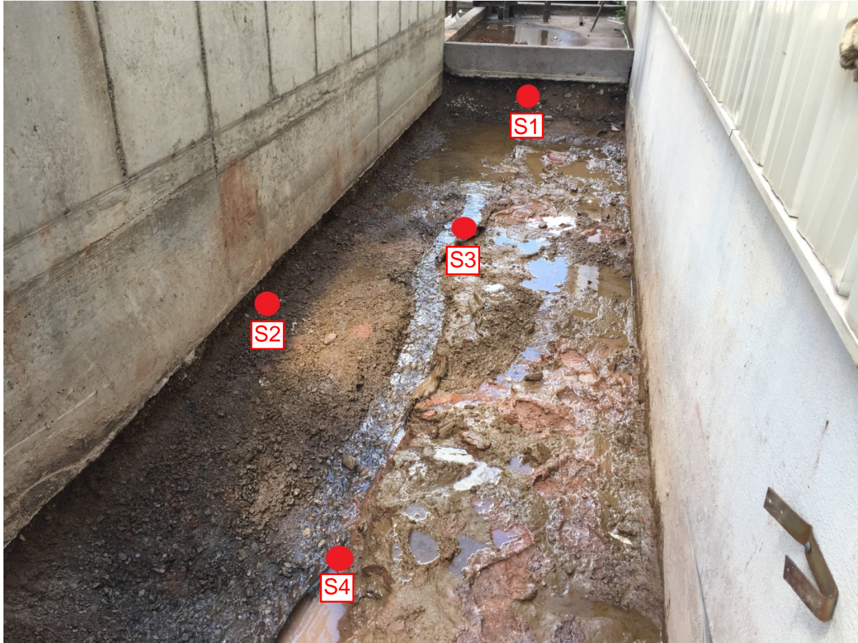
Photo 9: Looking east at the excavation and the sample locations for S1, S2, S3, and S4 (red dots).
