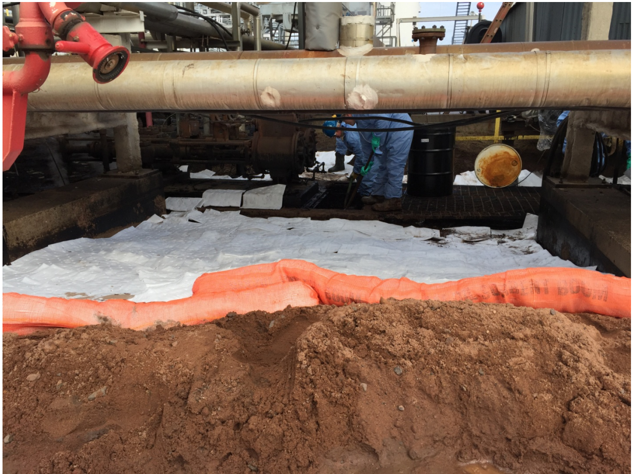
Photo 6: Looking north at the cleanup effort. As mentioned in Photo 2, a sand dam and absorbent booms were placed along the edges of the road to prevent further storm water from entering the site. Absorbent pads were placed on the excavated soil to soak up any potential contaminants that may have been missed after the initial excavation.
