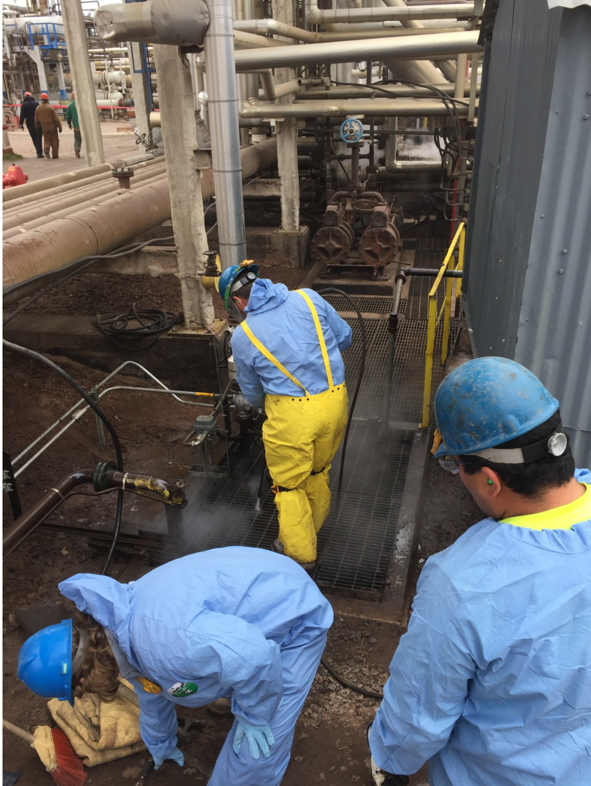
Photo 7: Looking west at the cleanup effort. In addition to soil removal, all contaminated surfaces were cleaned as well, which can be seen here. Steam pressure washers were used in combination with soap and hand tools to clean the affected surfaces.
