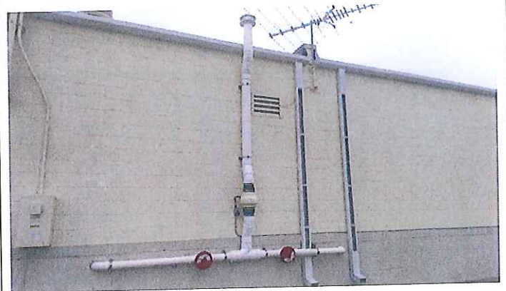
4. View of the PVC piping mounted on the exterior wall of the Village Clean facility. ...
