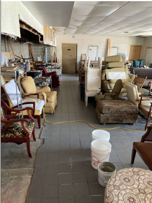
Title: Village Clean - View of Indoor Soil Cap building floor slab and tiles, no repairs needed
