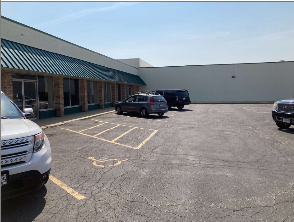
Title: Village Clean - View of Parking Lot Soil Cap, soil cap needs repair
