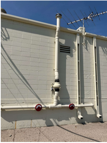
Description: Fan, valves, and discharge
