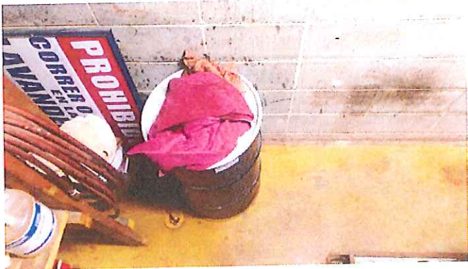
3. View of the interior concrete floor of the Village Clean facility behind the dry cleaning machine....
