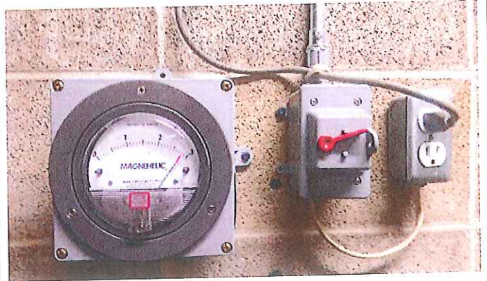
2. View of the Magnehelic pressure gage mounted behind the dry cleaning machine. The pressure gage is reading 2.5 inches of water.
