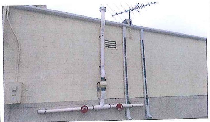
4. View of the PVC piping mounted on the exterior wall of the Village Clean facility. ...
