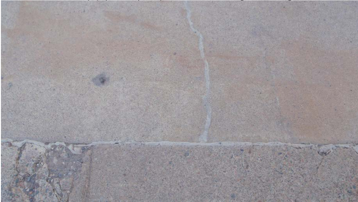
Photo 2 – concrete cap (top e/4 of photo) shown with caulking around edges and in crack.
