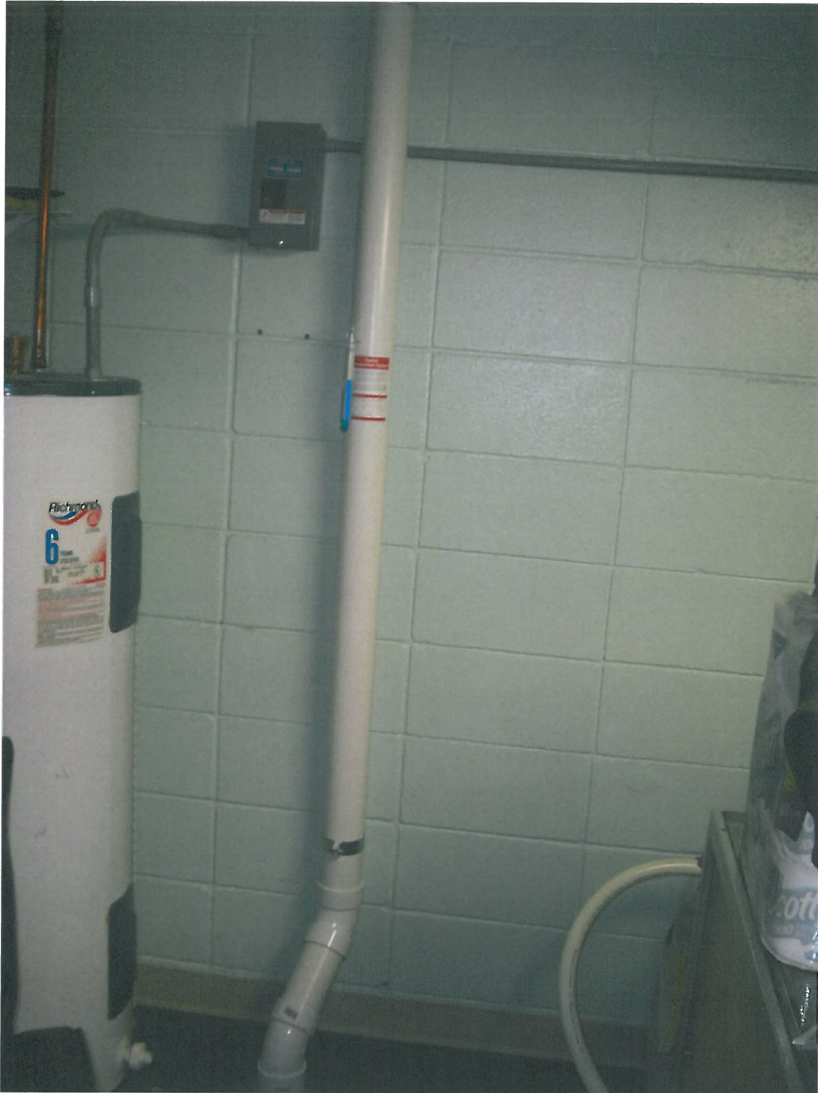
Viewing the sub-slab depressurization system installed on April 19, 2012 at the former Exotic Nails property. Note blue anemometer near the top of the picture.
