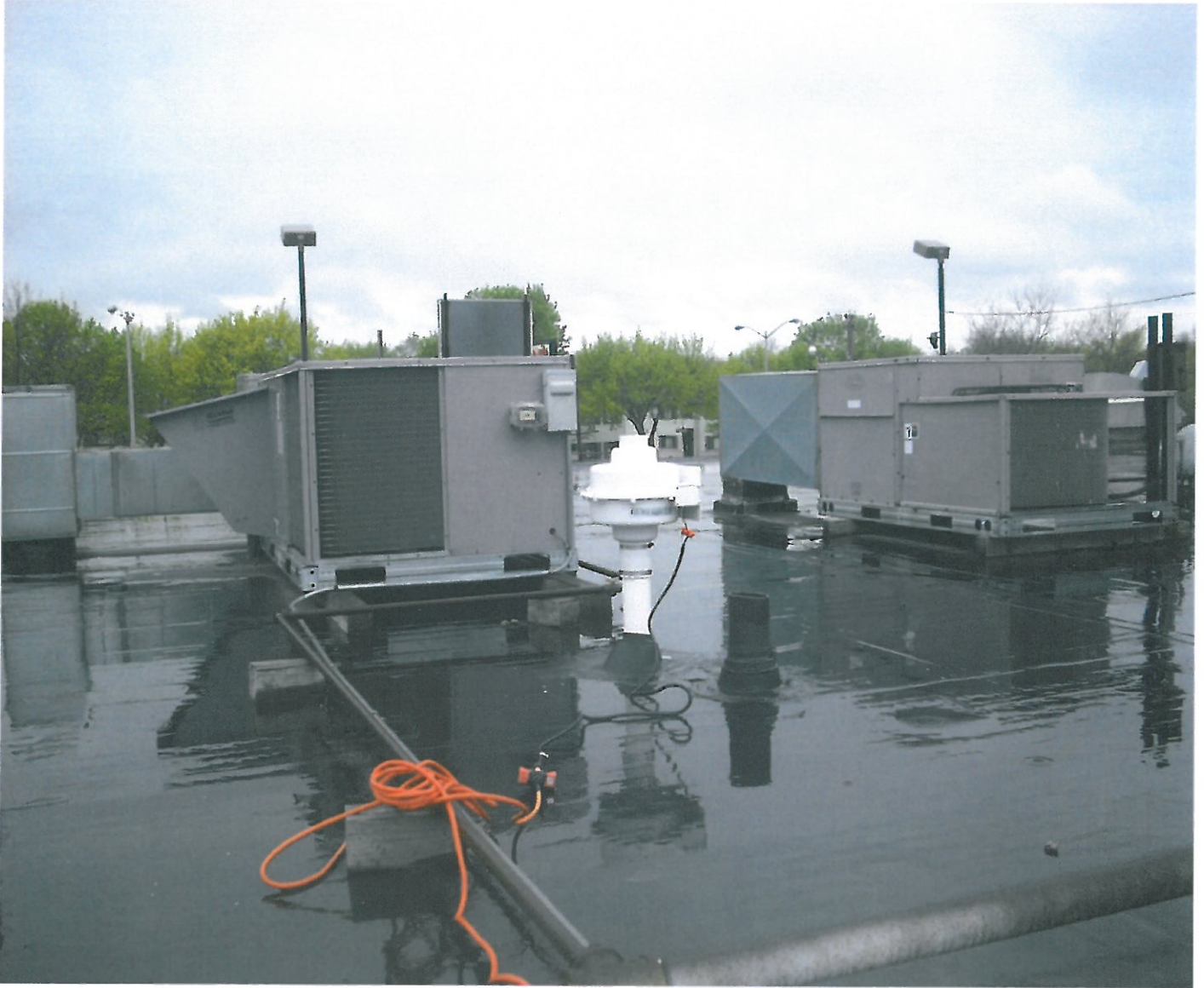
Viewing the roof penetration and fan placement at the former One-Hour Martinizing. The electrical wiring shown was temporary to test the functionality of the system. An electrician properly wired the system at a later date.
