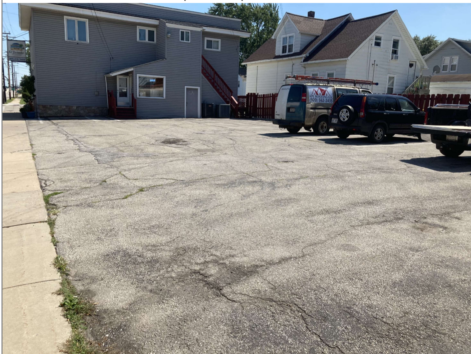
Title: 9/1/2022 - Looking SE toward building. Asphalt cap in place and in fair condition.
