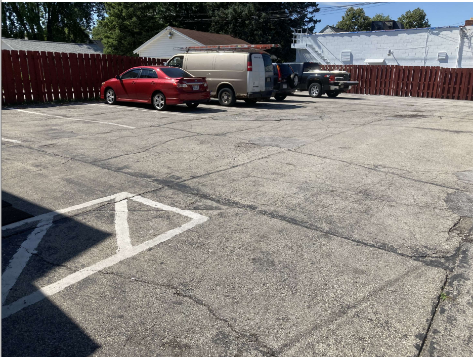
Title: 9/1/2022 - Looking W to west property corner across asphalt cap. Asphalt patch and tar filled cracks evident.
