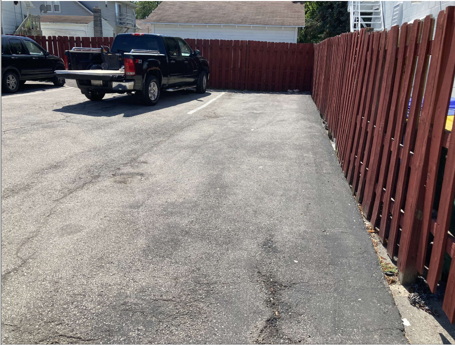
Title: 9/1/2022 - Looking SW along property line. Asphalt cap in place and in fair condition.
