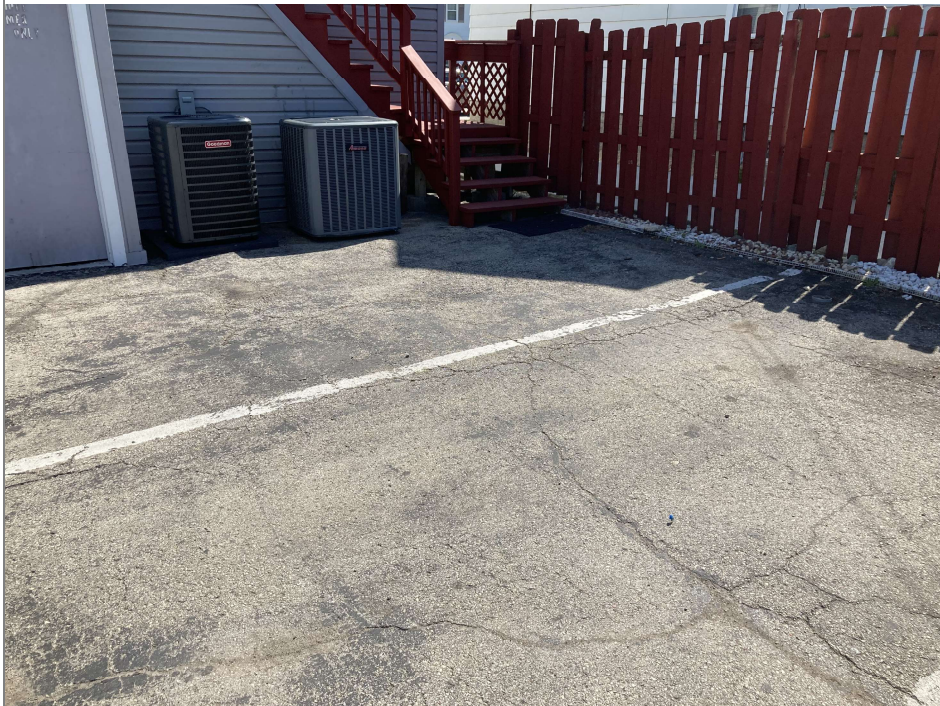
Title: 9/1/2022 - Looking S toward SW corner of building. Asphalt cap in place and in fair condition.
