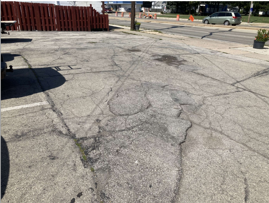
Title: 9/1/2022- Looking NW toward W Mason St across asphalt cap parking lot. Asphalt patch & tar filled cracks evident.
