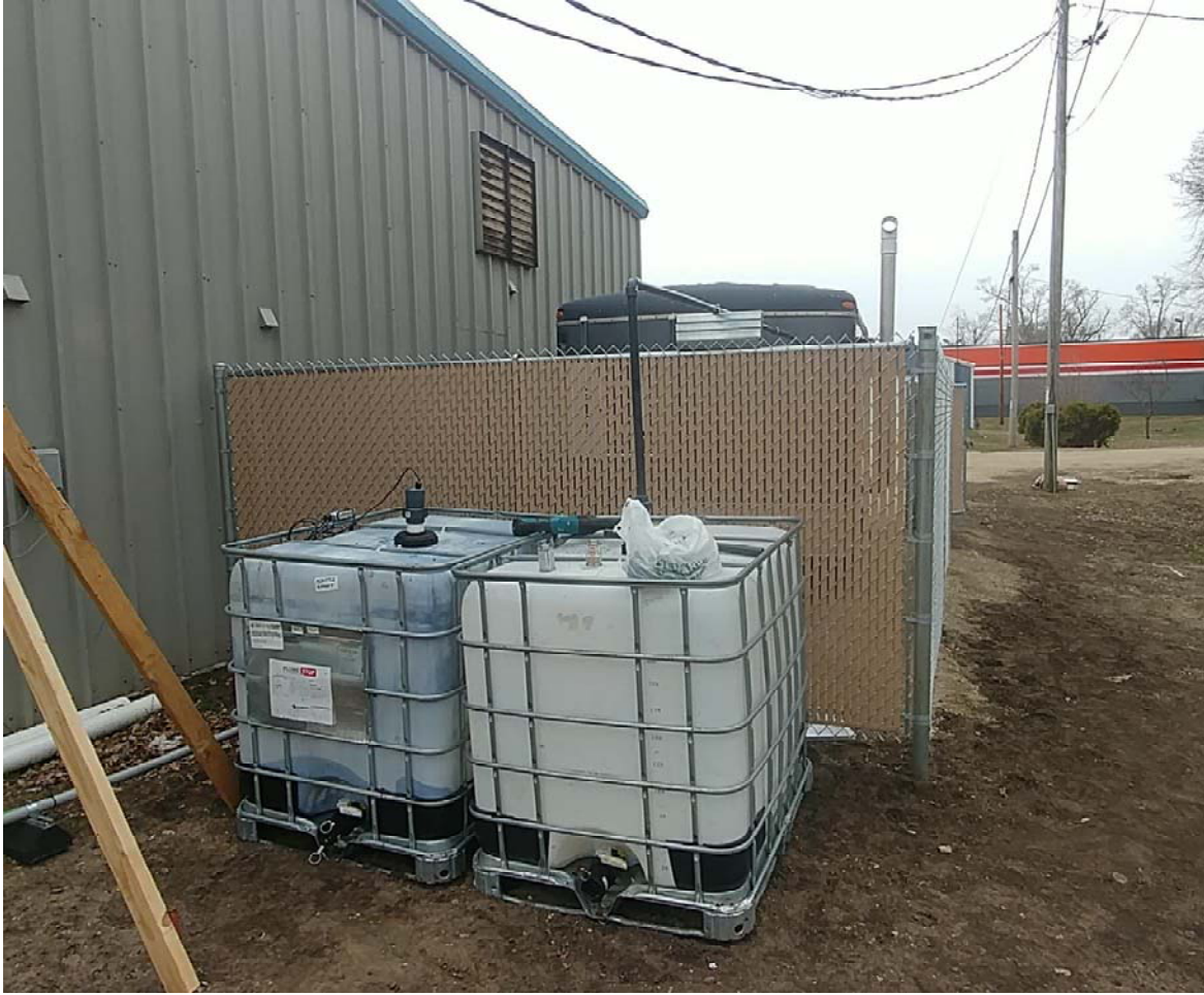
Installation complete, including security fence and storage tanks, facing south.
