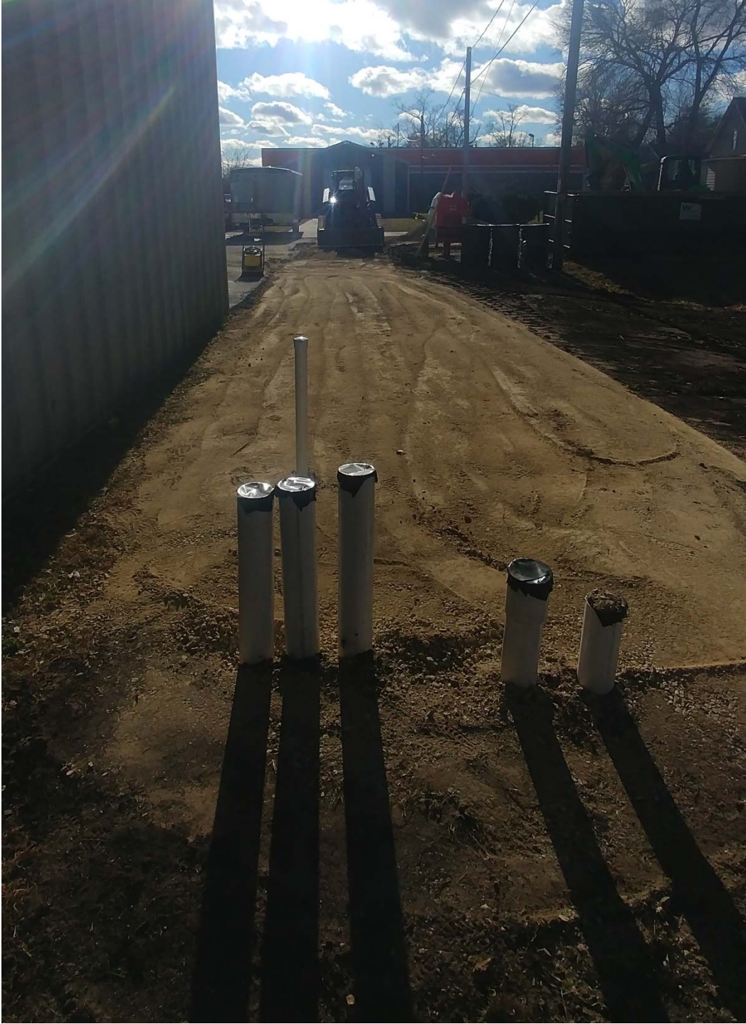
Conveyance line terminations and gravel pad for equipment trailer, facing south.
