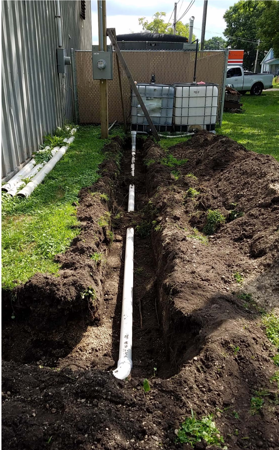
Installation of water discharge piping, facing south from northwest corner of building.
