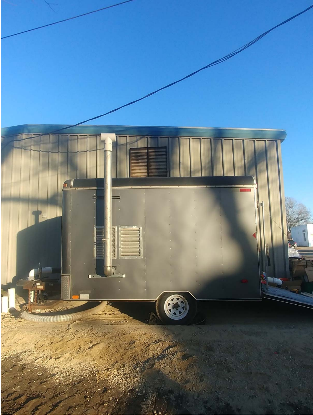
SVE equipment trailer in final position, facing east.
