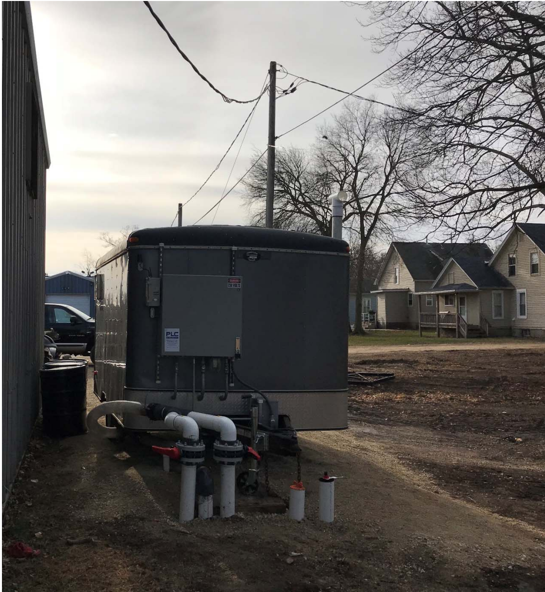
Conveyance piping connections to SVE equipment trailer (in progress), facing south.
