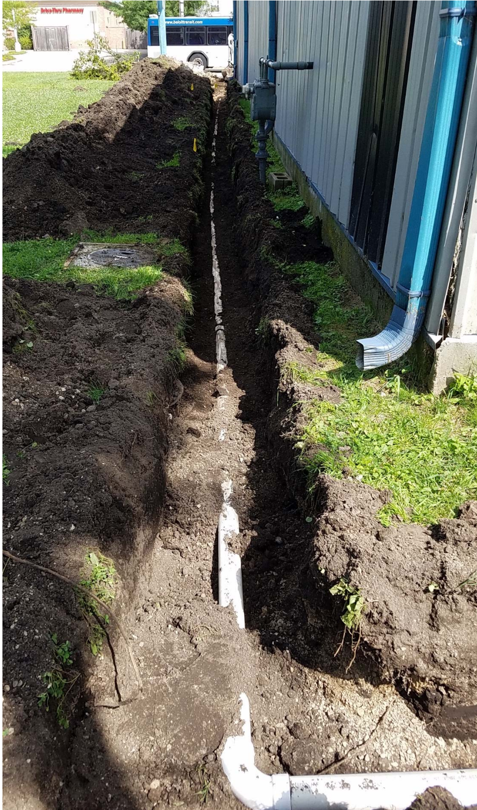
Installation of water discharge piping, facing east from northwest corner of building.
