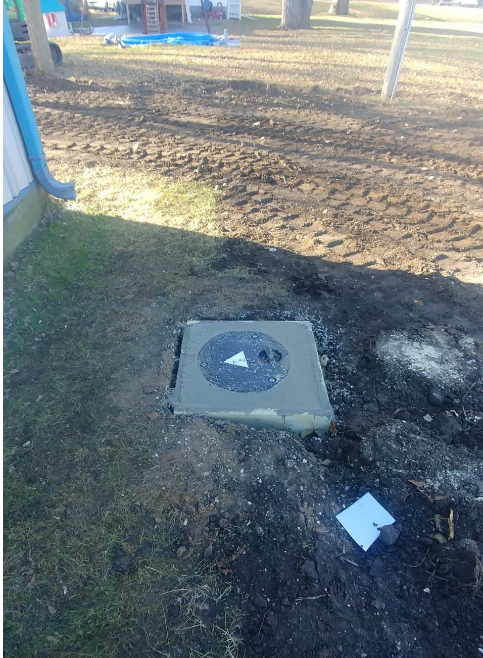
Typical extraction well vault in concrete pad.
