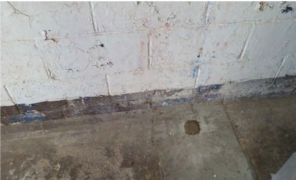
Photo 22: West wall of dry cleaning building and former location of SVE-3 pipe.
