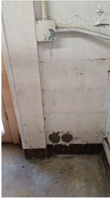
Photo 15: Patch at southwest corner of dry cleaning building where SVE lines entered building
