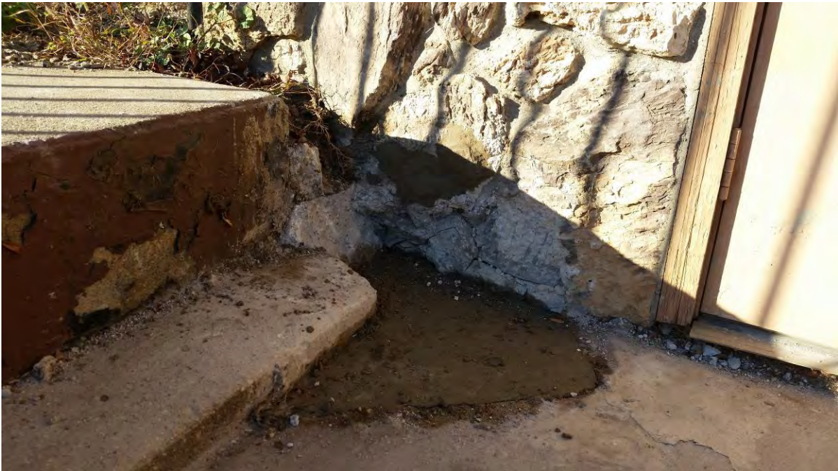
Photo 16: Patch in southwest corner of dry cleaner wall and pavement where SVE piping entered building
