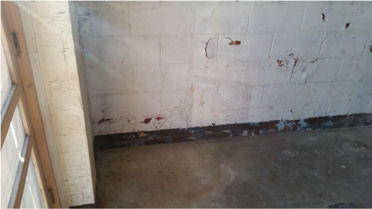
Photo 21: Southwest corner of dry cleaning building and former location of SVE knockout tank
