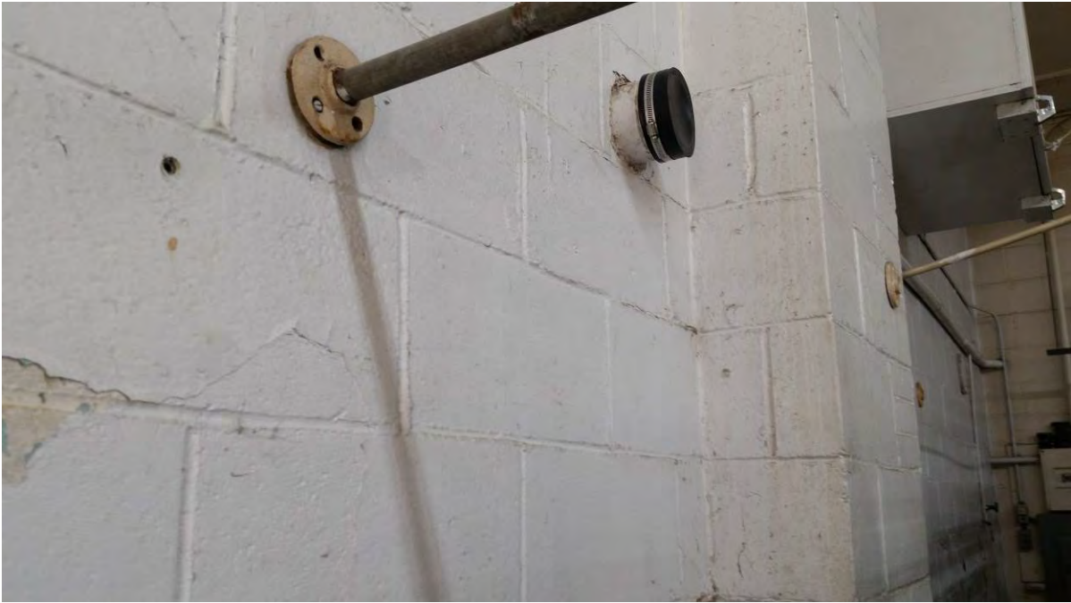
Photo 17: Capped pipe where SVE exhaust line exited west wall of dry cleaning building
