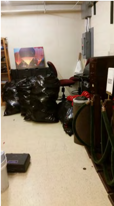
Photo 14: Abandoned First National Bank sub-slab port (right side of photo)
