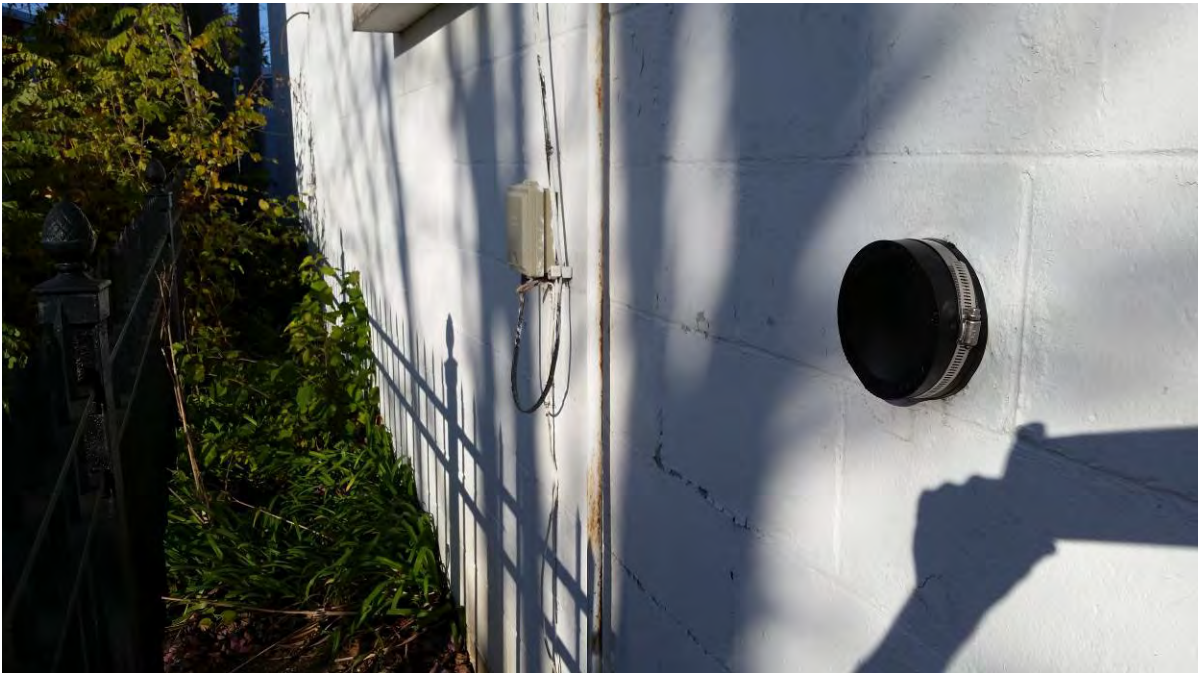
Photo 18: West wall of dry cleaning building and capped pipe where SVE exhaust line exited the building. Pipe was present prior to SVE system construction.
