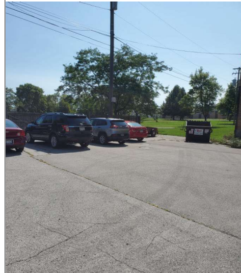
Title: East portion of asphalt cap replaced by City of Two Rivers in 2014.
