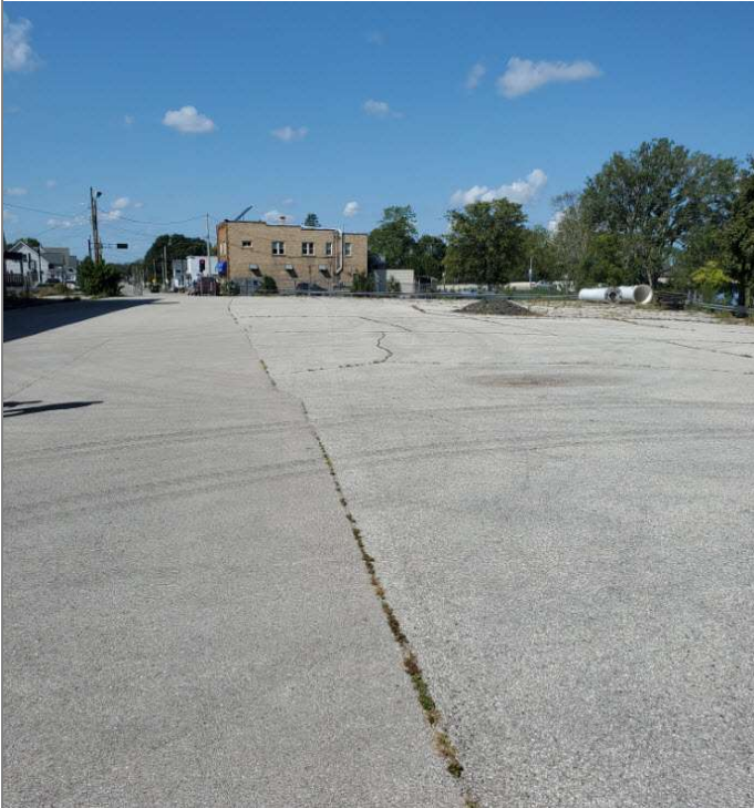
Title: Required asphalt pavement cap (right side of photo), easement area where asphalt was replaced after utility work in 2014 (left side of photo), looking west.
