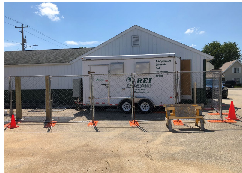
SVE system for Nail Boutique on site awaiting electrical service connection
