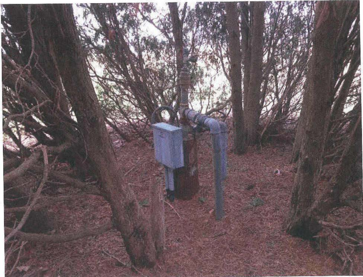
Photo 1 Groundwater Extraction Well
