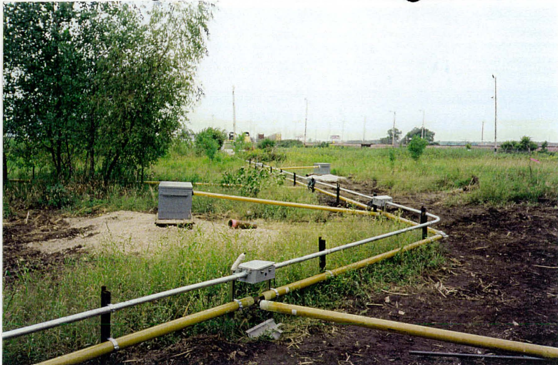
PHOTO #1: LATERAL AND HEADER PIPE TRANSFER LINES.
