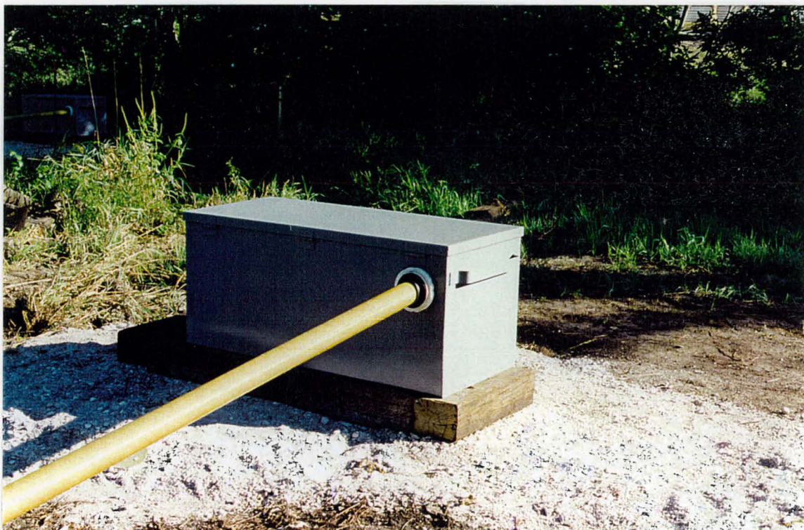
PHOTO #2: TYPICAL WELL VAULT AND TRANSFER PIPE.
