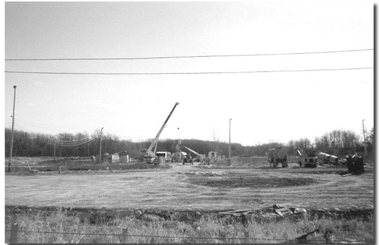
The LTTD equipment at the site was decontaminated, disassembled and removed earlier this year.
