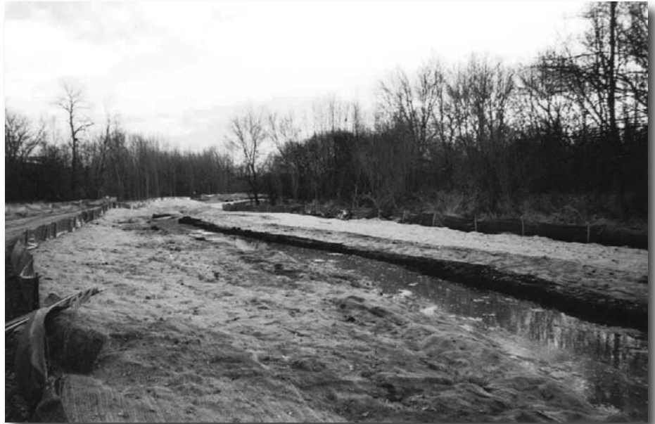
Work on segments 2 and 3 of the Little Menomonee River may look like this (segment 1) while they are being rerouted.
