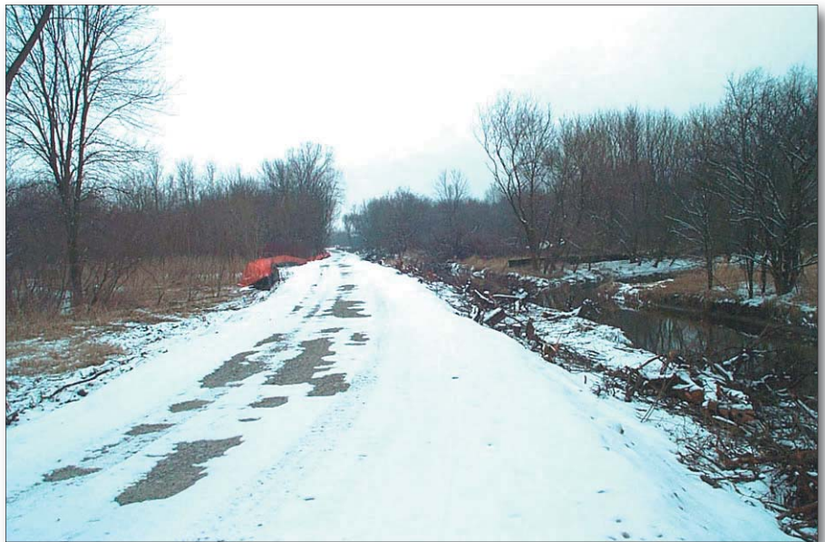
This newly built access road is being used to bring in heavy equipment for the creation of the new channel and wetlands south of Bradley Road.
