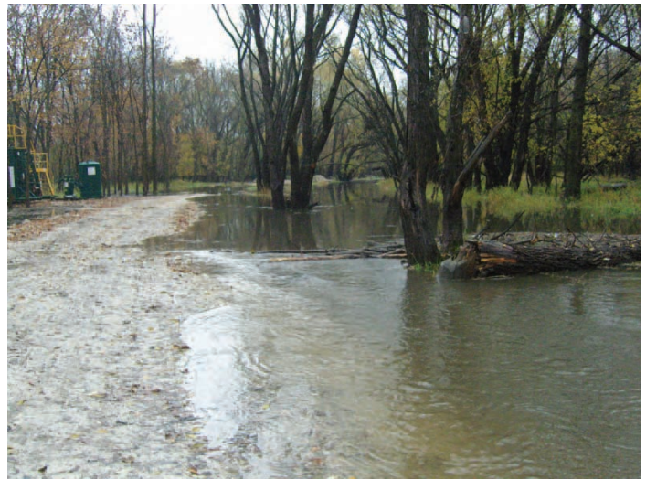
Flooding in the Little Menomonee River put the dredging project three to four weeks behind schedule.
