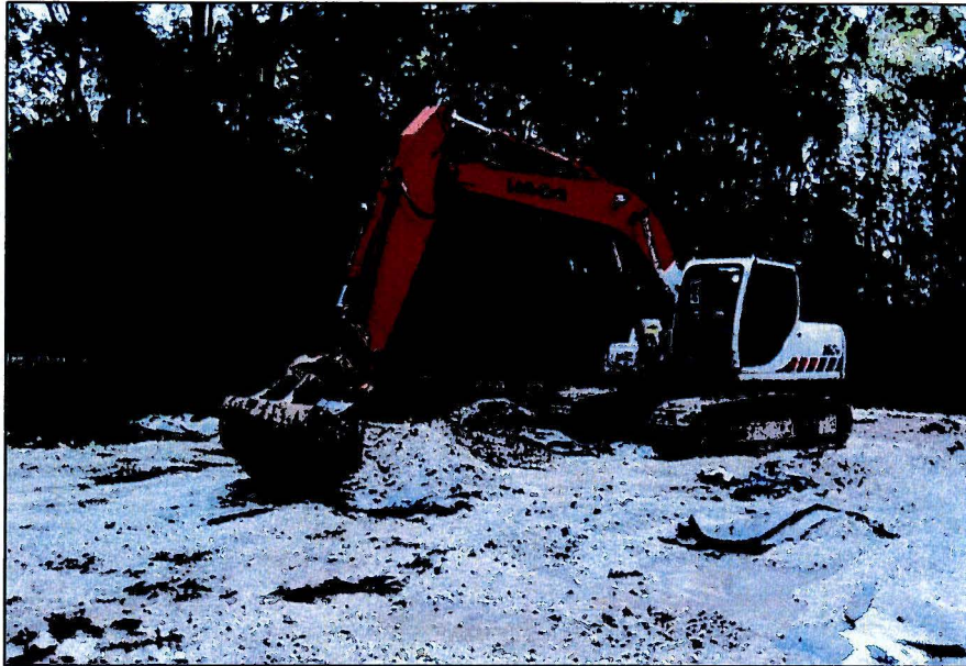
Photograph No.: 15 Photographer: Naren Babu Date: 9/29/2009 Subject: Back Hoe removing gravel and geofabric liner from access roads.
