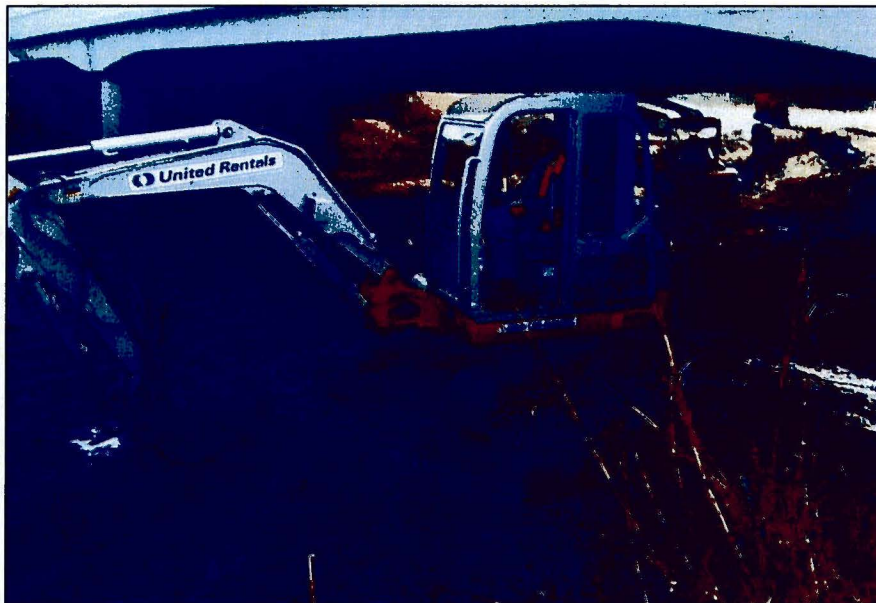
Photograph No.: 14 Photographer: Naren Babu Date: 11/10/2009 Subject: Excavator removing contaminated sediments underneath Appleton Avenue bridge.
