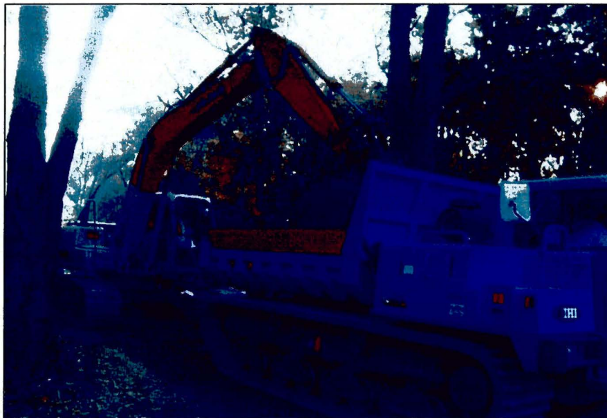
Photograph No.: 8 Photographer: Naren Babu Date: 9/10/2009 Subject: Back Hoe loading Scubic yard truck with sediments from Work Area #8.
