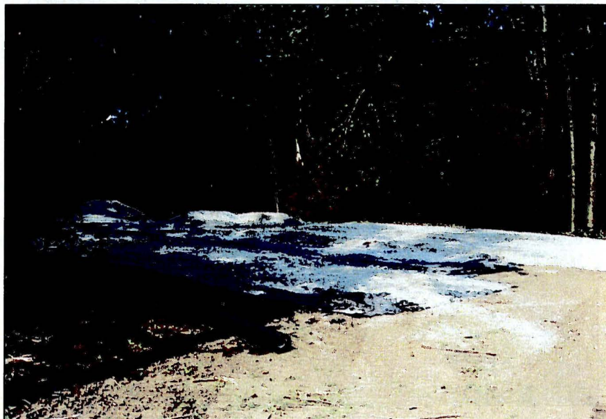
Photograph No.: 4 Photographer: Troy Thompson Date: 8/15/2009 Subject: for pumps was constructed with soil, gravel and geofabric along the Little e river at Silver Spring Access area.
