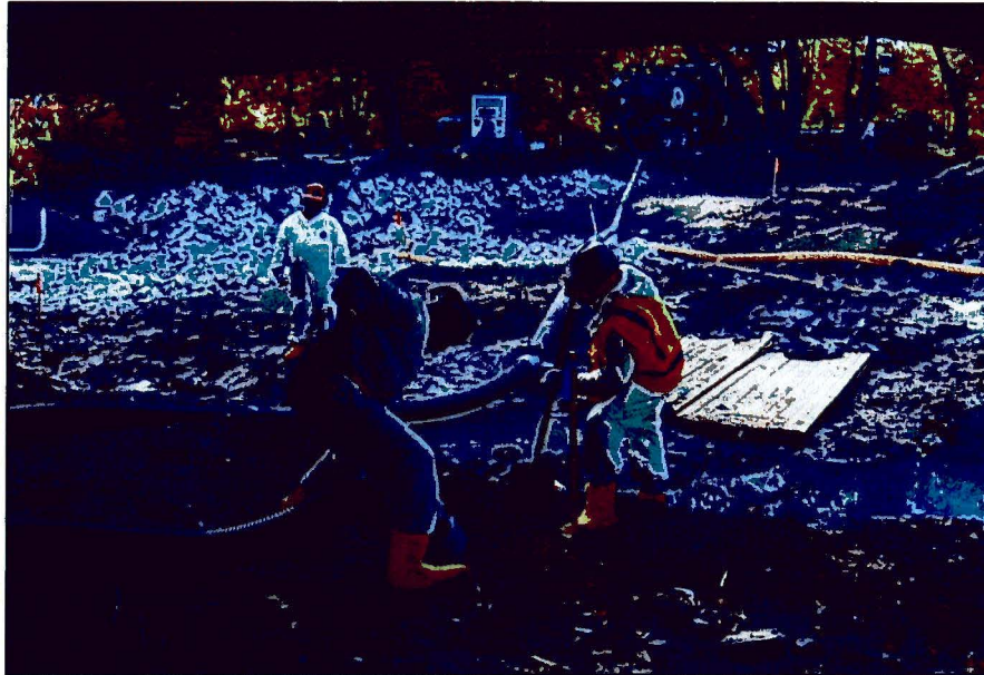
Photograph No.: 11 Photographer: Troy Thompson Date: 9/17/2009 Subject: ERRS removing sediments with Vacuum hoses at Work Area #13 under Silver Spring Drive Bridge.
