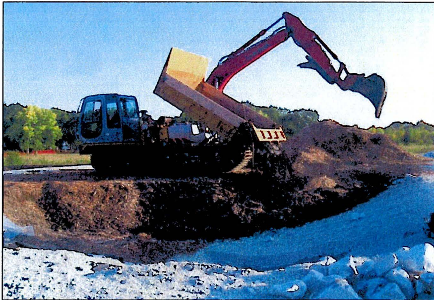
Photograph No.: 9 Photographer: Naren Babu Date: 9/11/2009 Subject: 5 cubic yard truck unloading sediments at the sediment dewatering pad on 107 th Street access area.
