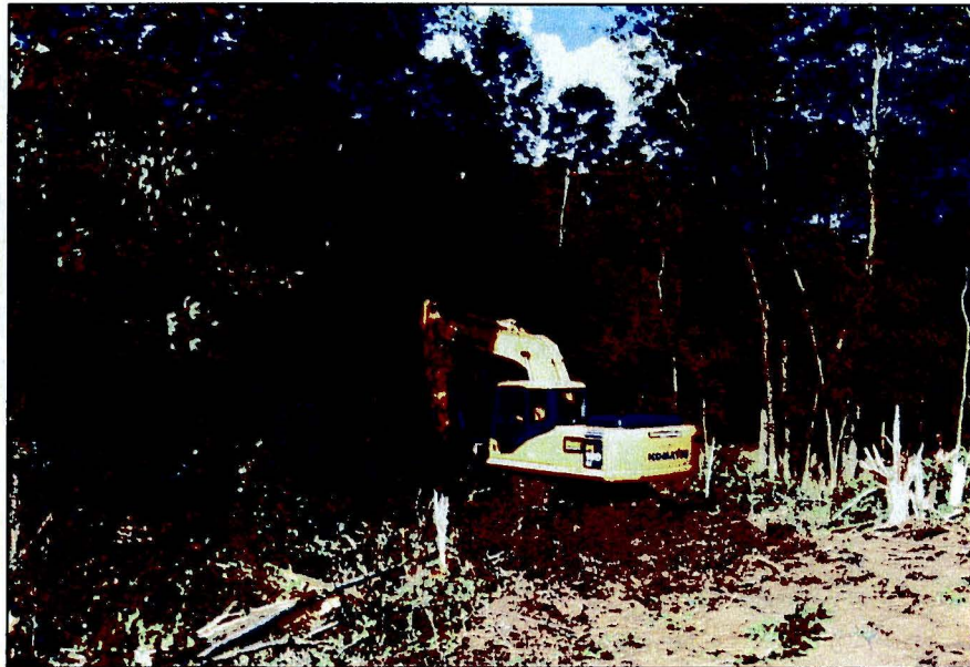
Photograph No.: 2 Photographer: Troy Thompson Date: 8/10/2009 Subject: ERRS clearing the trees with a back hoe for access roads.
