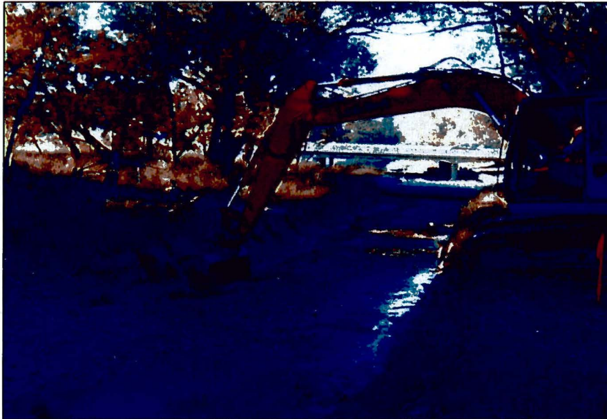
Photograph No.: 7 Photographer: Naren Babu Date: 09/11/2009 Subject: Excavator removing contaminated sediments from the river at the southern segment of Reach 4/5.
