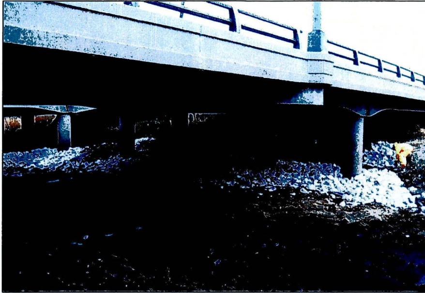
Photograph No.: 17 Photographer: Naren Babu Date: 11/17/2009 Subject: Rip raps were placed around the footings of the bridges for stabilization and erosion control.
