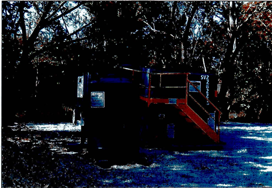
Photograph No.: 5 Photographer: Troy Thompson Date: 8/24/2009 Subject: General view of Frac tank and water treatment equipment on the staging pad.
