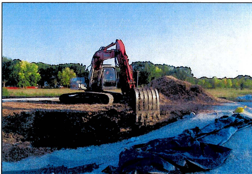
Photograph No.: 10 Photographer: Naren Babu Date: 9/11/2009 Subject: Back Hoe mixing the sediments with saw dust at the sediment dewatering pad on 107 th Street access area.
