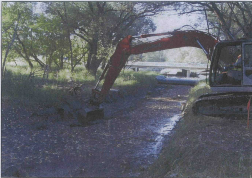
Photograph No.: 6 Photographer: Troy Thompson Date: 09/11/2009 Subject: Excavator removing contaminated sediments from the river at the southern segment of Reach 4/5.
