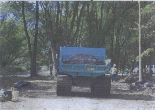
Excavated sediment being hauled away at Reach 4/5 at Little Menomonee River (August 31, 2009)
