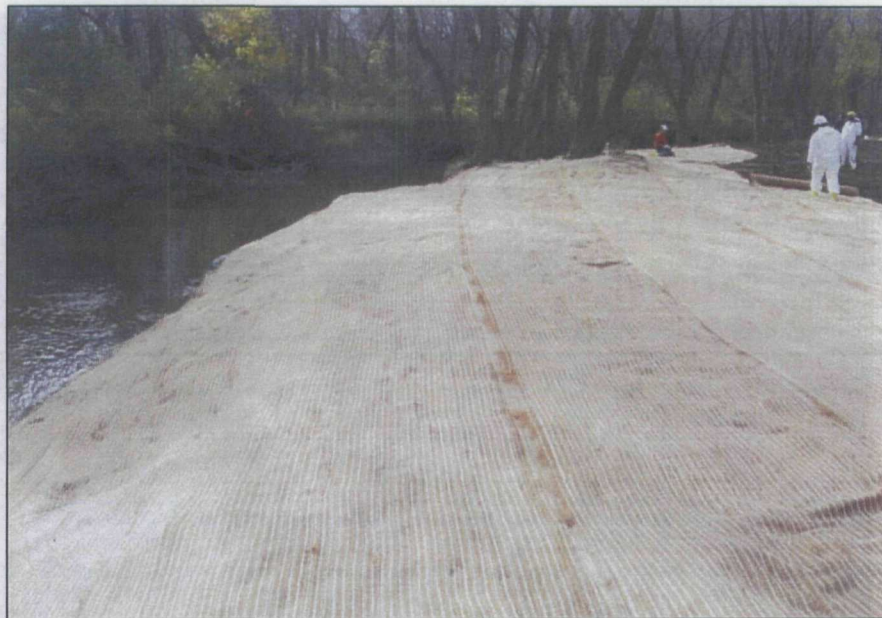
Photograph No.: 8 Photographer: Naren Babu Date: 10/28/2009 Subject: Disturbed areas along the Little Menomonee river during sediment removal were regraded, seeded and covered with coir mats for erosion control.
