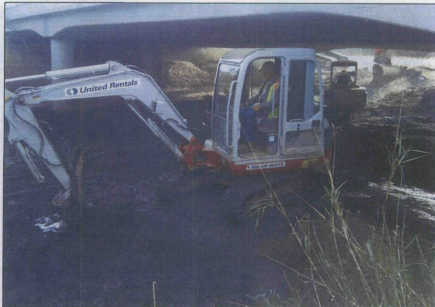
Photograph No.: 7 Photographer: Naren Babu Date: 11/10/2009 Subject: Excavator removing contaminated sediments underneath Appleton Avenue bridge.
