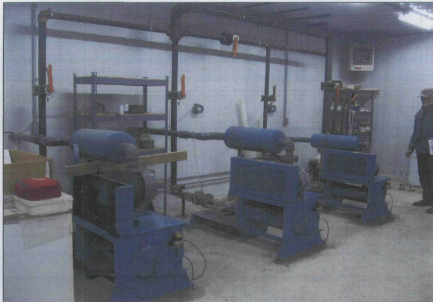
Photograph No.: 4 Photographer: Naren Babu Date: 10/09/2009 Subject: View of the three units inside the groundwater treatment system building.
