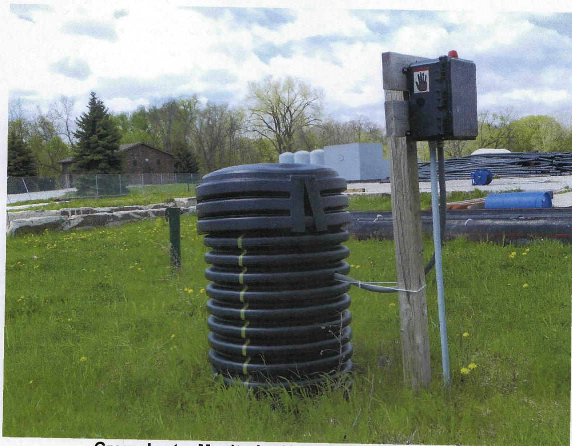
Groundwater Monitoring/ Interceptor Trench Sump
