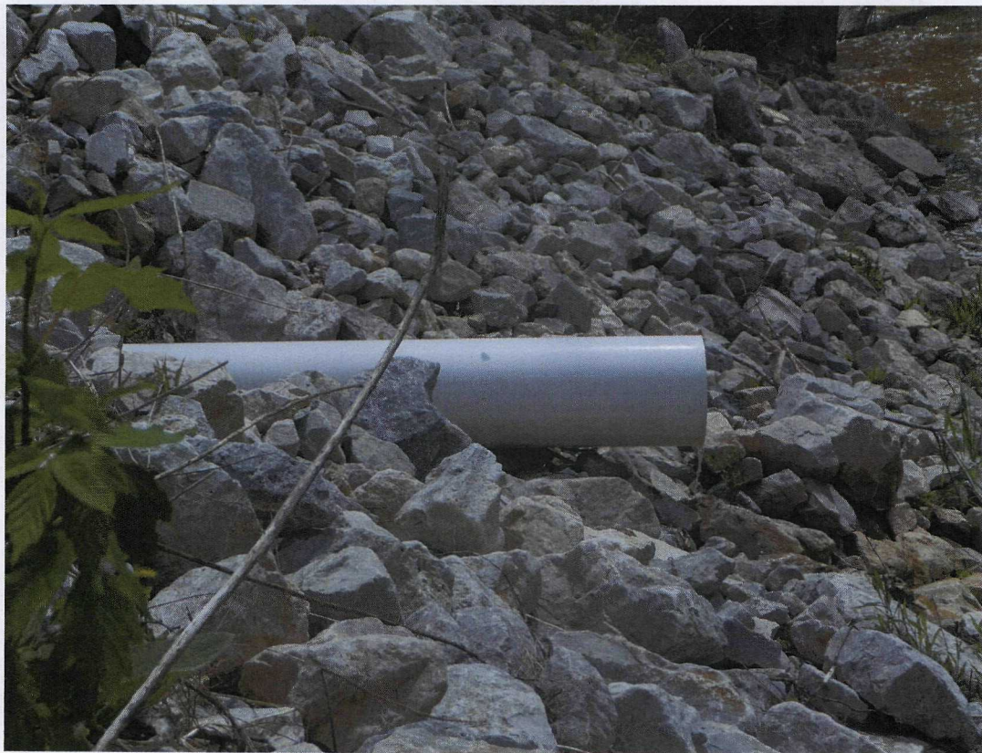
Discharge wastewater treatment plant
