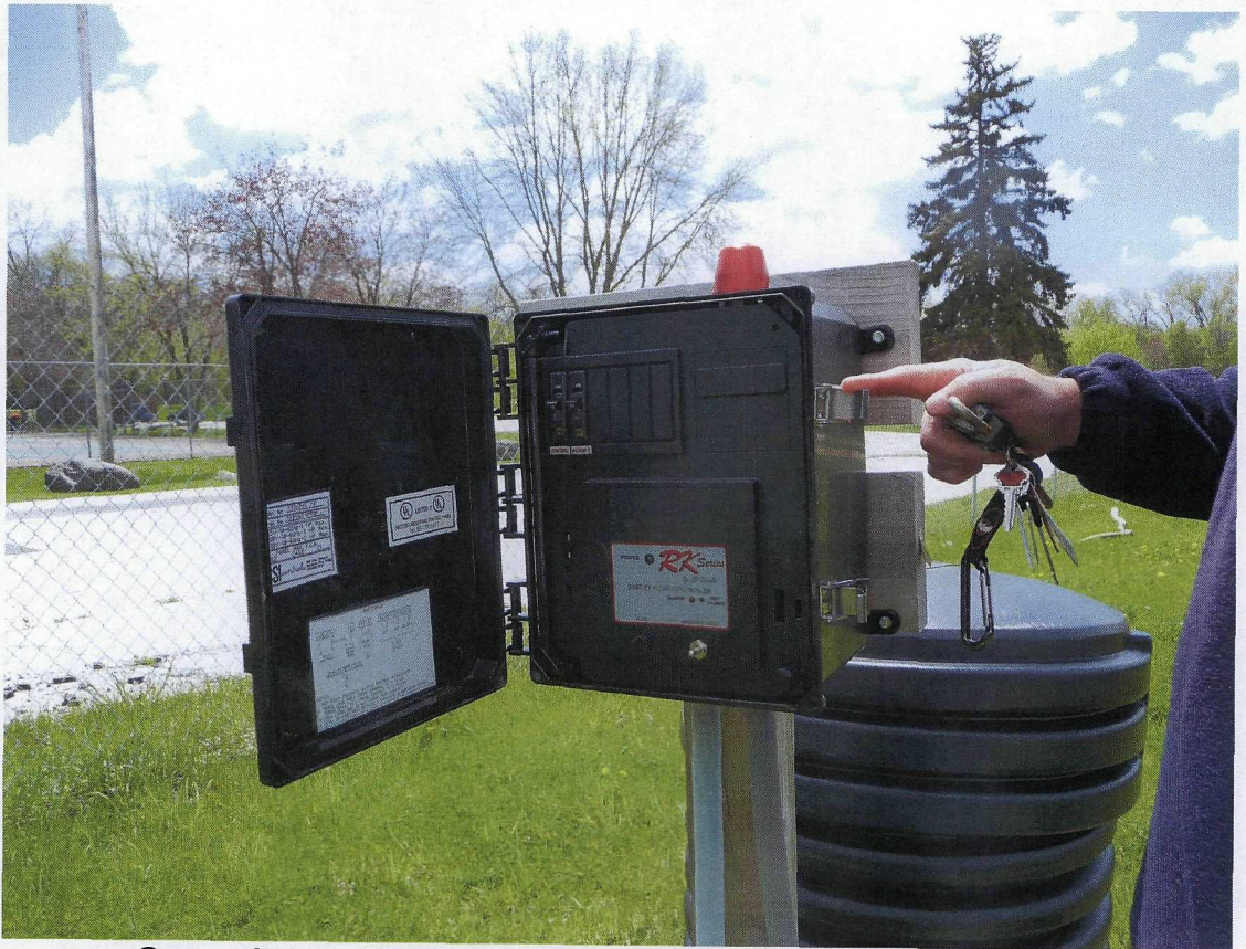
Groundwater Monitoring/ Interceptor trench control panel
