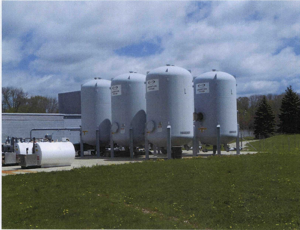
Waste water treatment plant at former Tecumseh property
