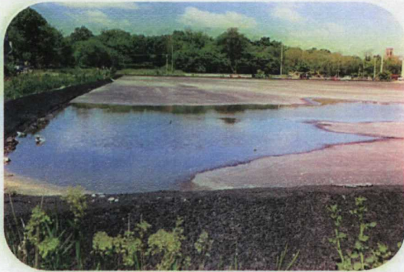
Water ponding at dewatering pad at former Tecumseh plant
