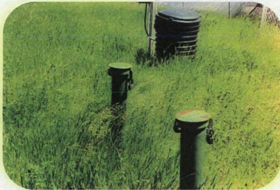
Sump pump for groundwater interception trench and monitoring wells MW-9 and MW-10
