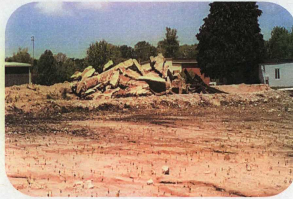
Construction debris at Maryland avenue dewatering pad
