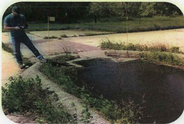
Water ponding at sump in the Former Tecumseh plant dewatering pad
