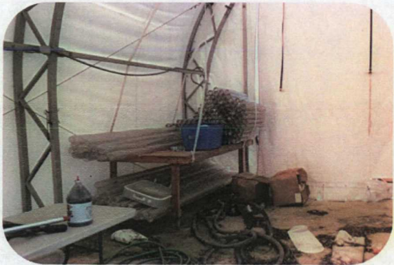
Interior of temporary building containing waste water treatment plant equipment
