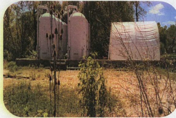
Waste water Treatment plant at Maryland avenue dewatering pad
