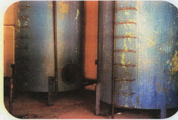
Oil separators at building in former Tecumseh plant
