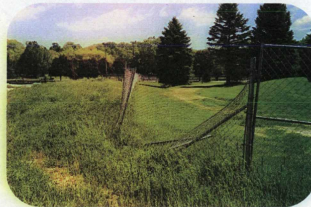
Damaged fence in north east corner of the former Tecumseh Plant Location
