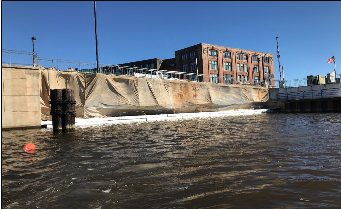
PHOTO NO. 11: View of the inaccessible area of the Inner Harbor (Grids 112 and 114) beneath the southern portion of the 8 th Street Bridge.
