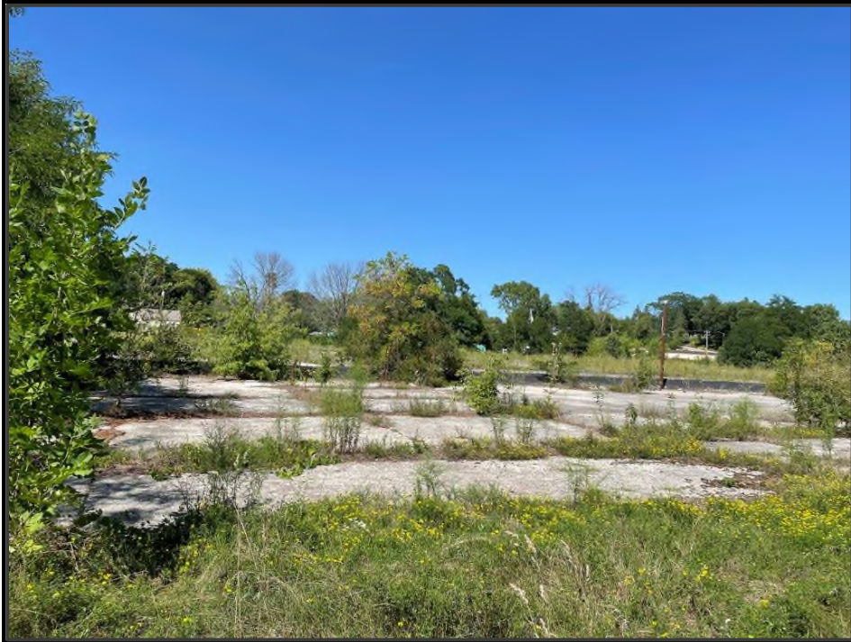
PHOTO NO. 17: View of pavement in the eastern portion of the Site.
