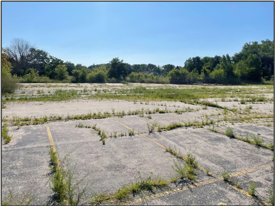
PHOTO NO. 22: View of pavement in the western portion of the Site.
