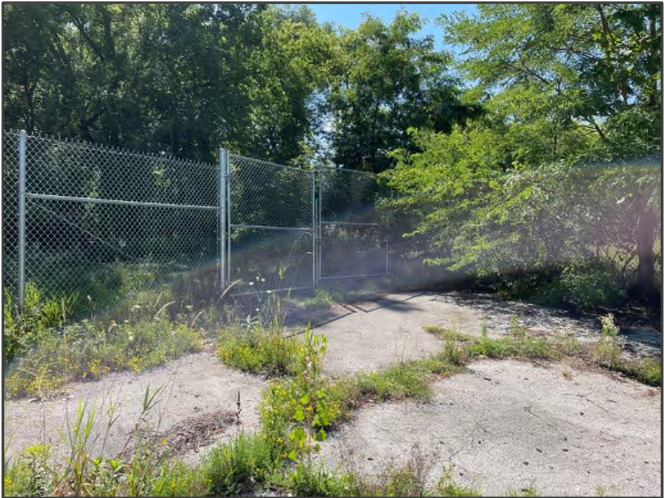
PHOTO NO. 14: View of fence along the south side of the Site.
