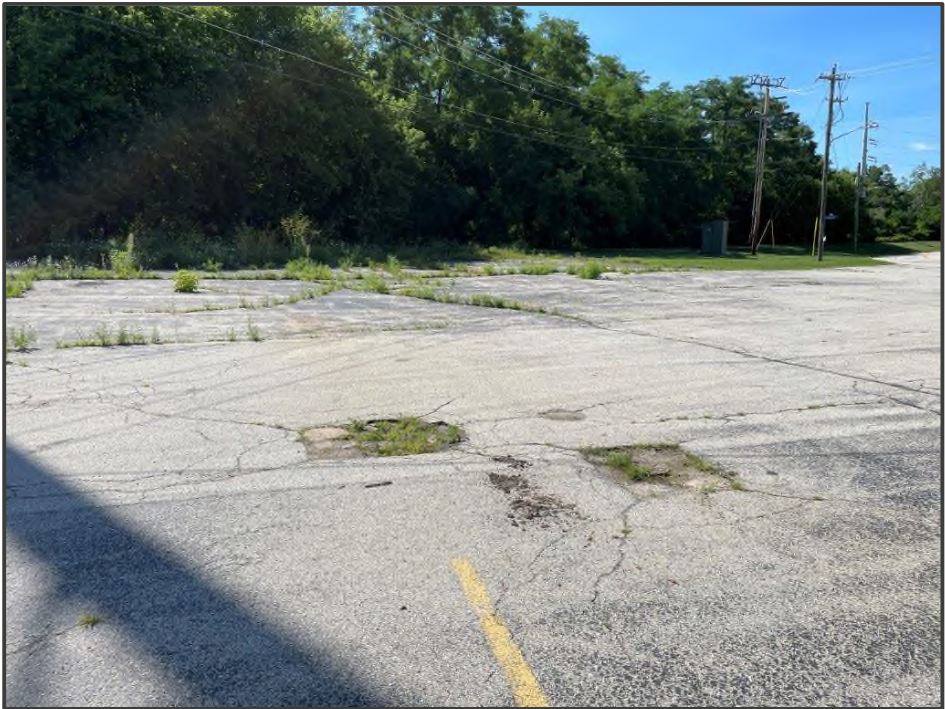
PHOTO NO. 20: View of pavement in the central portion of the Site.
