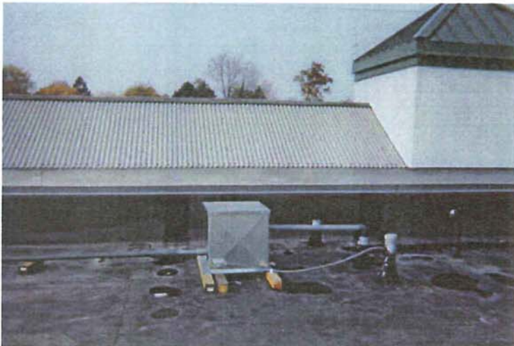
3. Vapor Mitigation System on the Roof.
