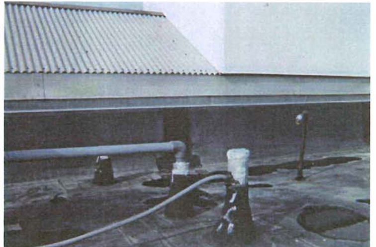
4. Plugged roof vents.
