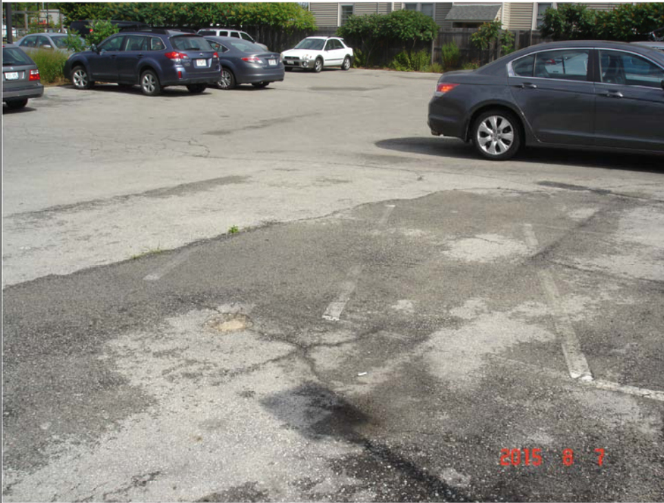
Title: Photo #3. Abandoned monitoring well visible (brownish circle) at the lower left of center of photo.
