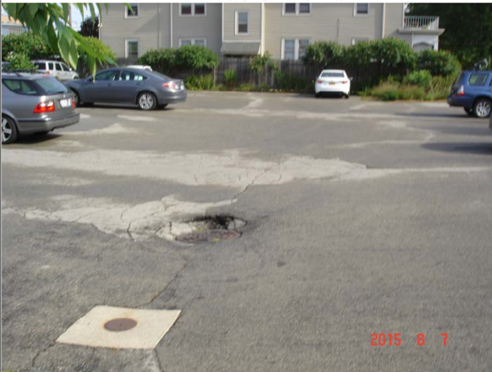
Title: Photo #2. Storm drain at the parking lot. This drain is not indicated in any map in the GIS Registry.
