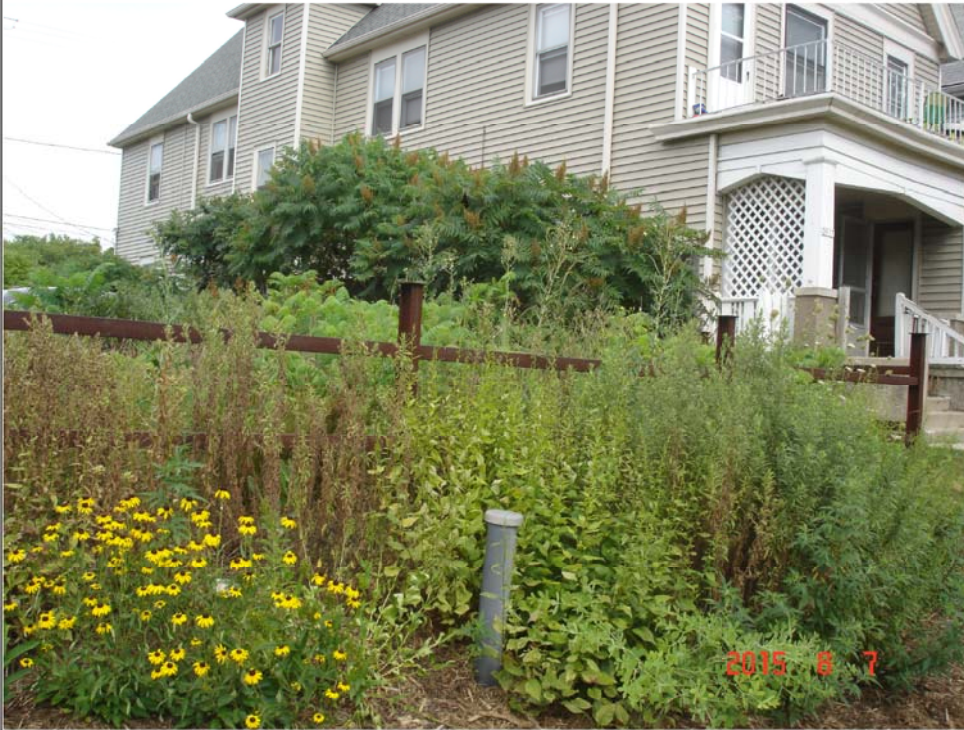
Title: Photo #5. Passive venting (stick-up) pipe near the sidewalk to the east of the parking lot
