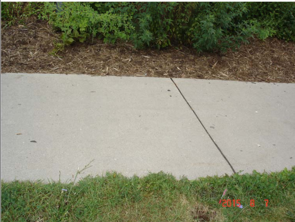
Title: Photo #6. Photo taken just on the other side of the sidewalk from the stick-up venting pipe. There is a freshly-placed hole in the grassy part. Hole is probably for a street sign.
