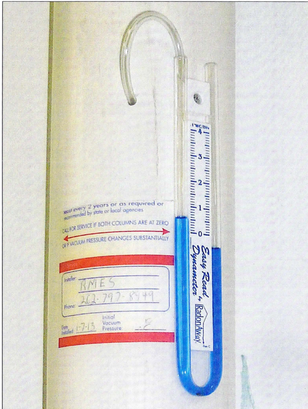
Manometer Installed on draw tube 3 as shown in Photo 3
