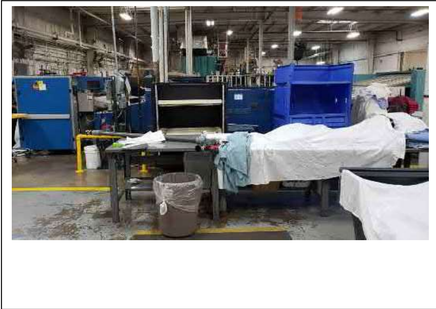
PHOTOGRAPH # 4 Taken on: 12/27/2021 Location/Direction: View of the concrete floor within southwest corner of the building.
