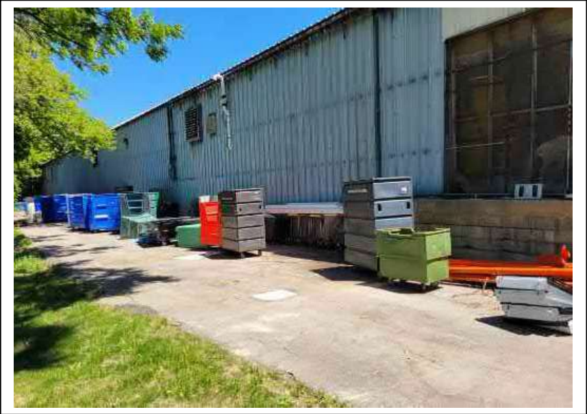
PHOTOGRAPH # 1 Taken on: 6/27/21 Description: View of engineered barrier along west side of building, facing northwest. Union Pacific Right-of-Way visible in the lower left (grass). White PVC vent pipe and blower associated with the Sub-Slab Depressurization System is visible in the center of the photo.
