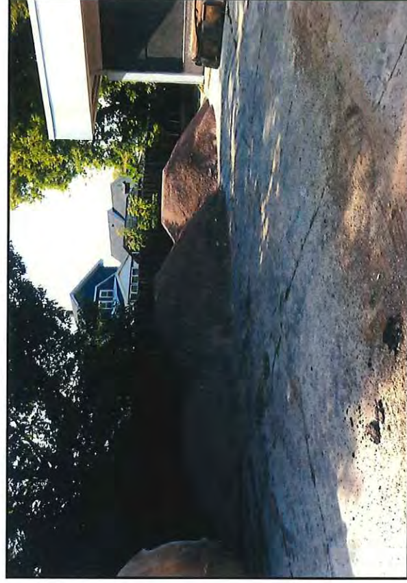
Contaminated 3/8" Stone - Stock Piled Onsite
