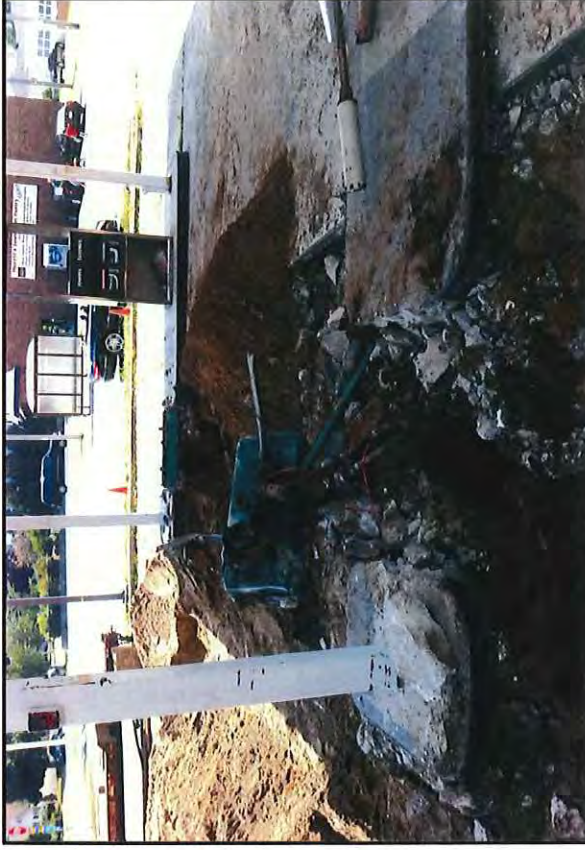
Tank Bed Location
