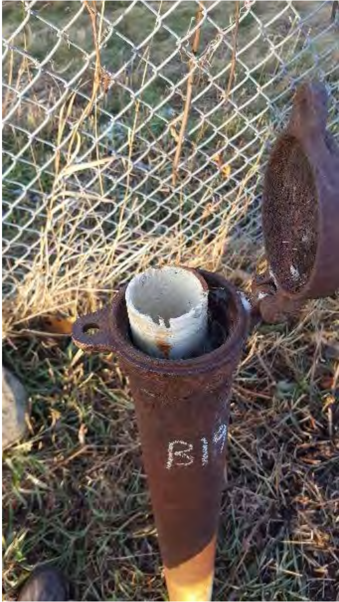
113. B-19, inside well, no cap damage to PVC, looking N
