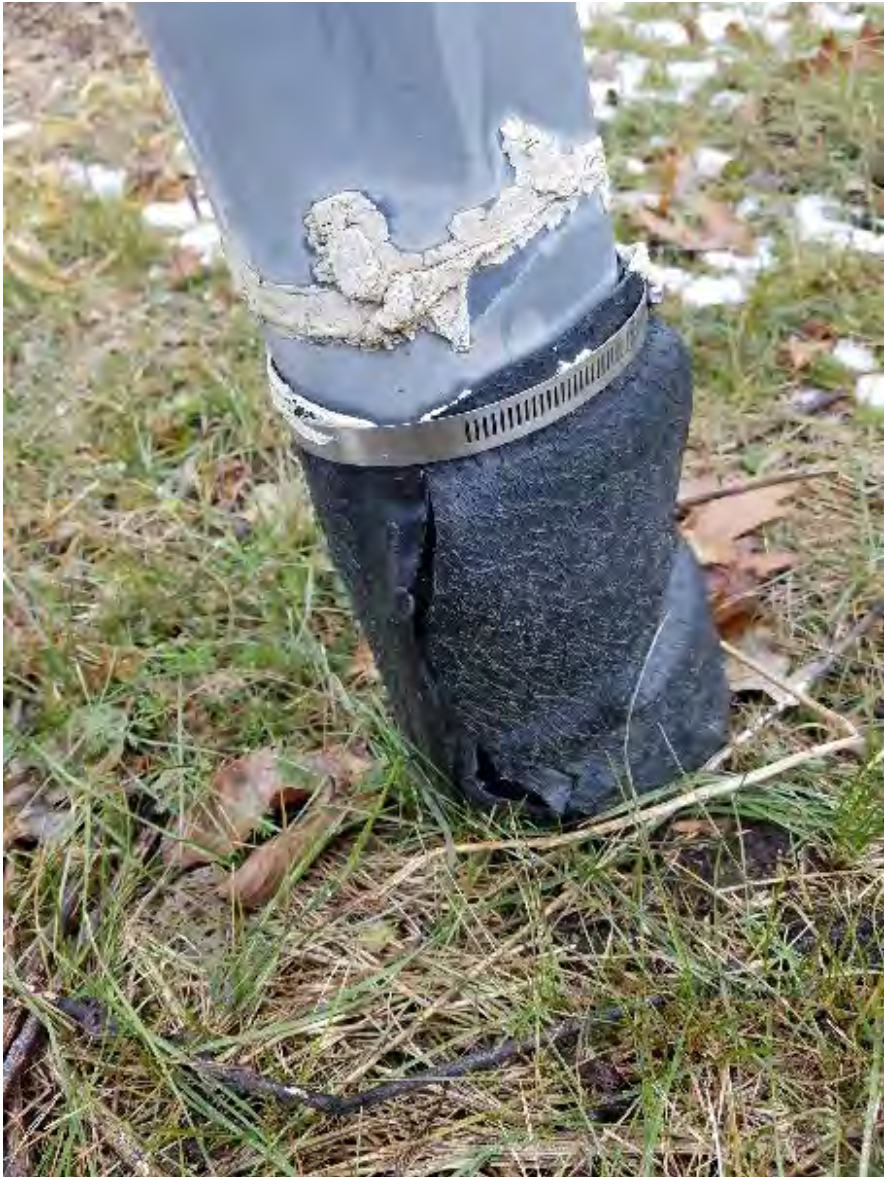
31. Unmarked GV by GP-9 damaged liner
