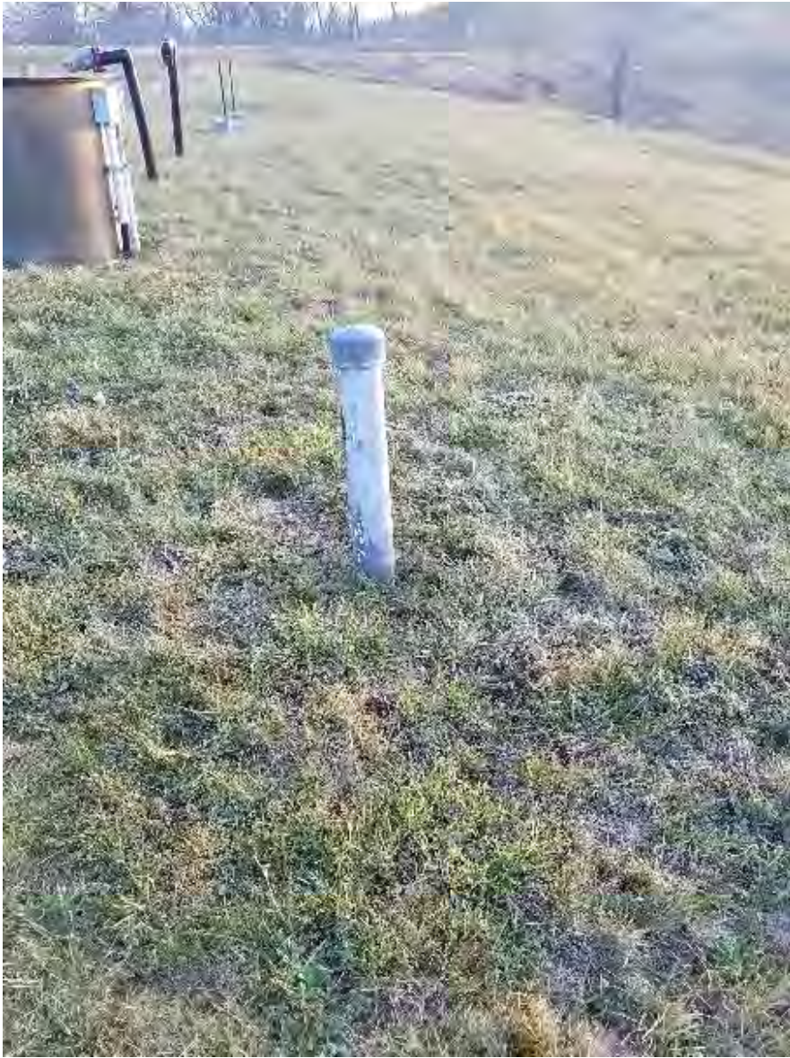
133. Possible LHW or GV, unmarked, looking S along leachate piping
