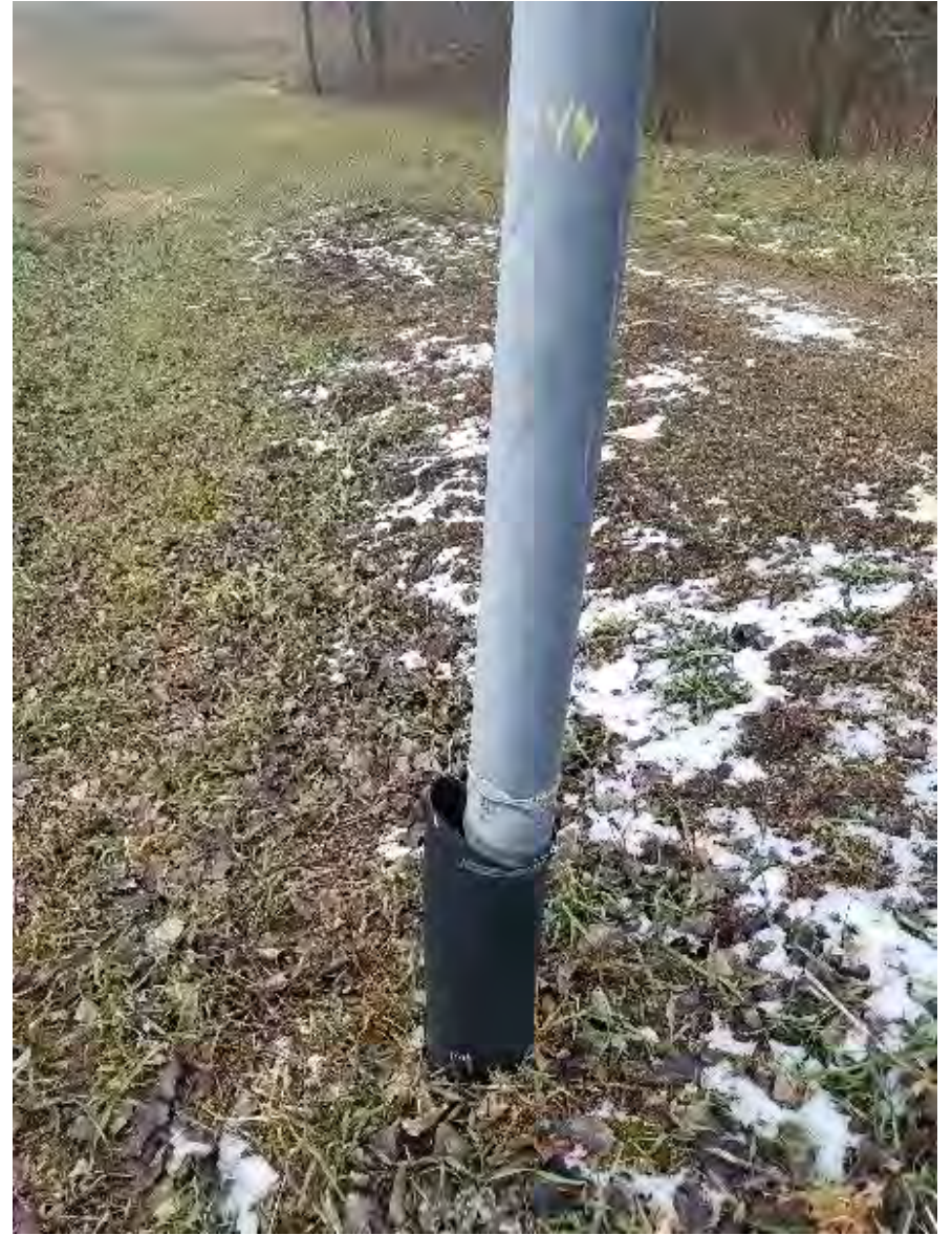
54. GV-44 looking E, hose clamp needs to be tightened
