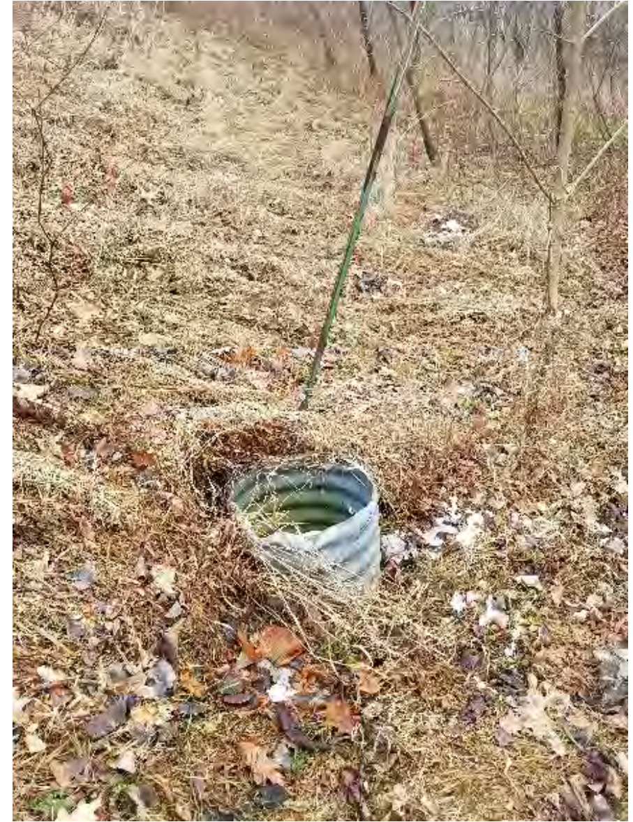
62. Unknown pipes in ground, not marked, N of B-96-17, looking S
