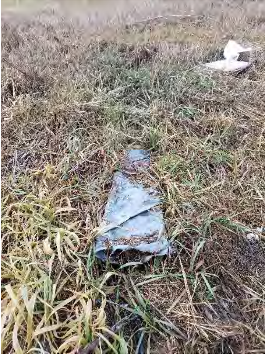
17. Damaged drain pipe, looking NE
