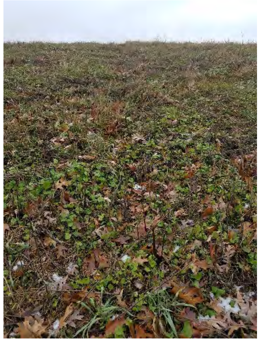
90. Slight erosion or tire tacks, looking S uphill towards GV-11
