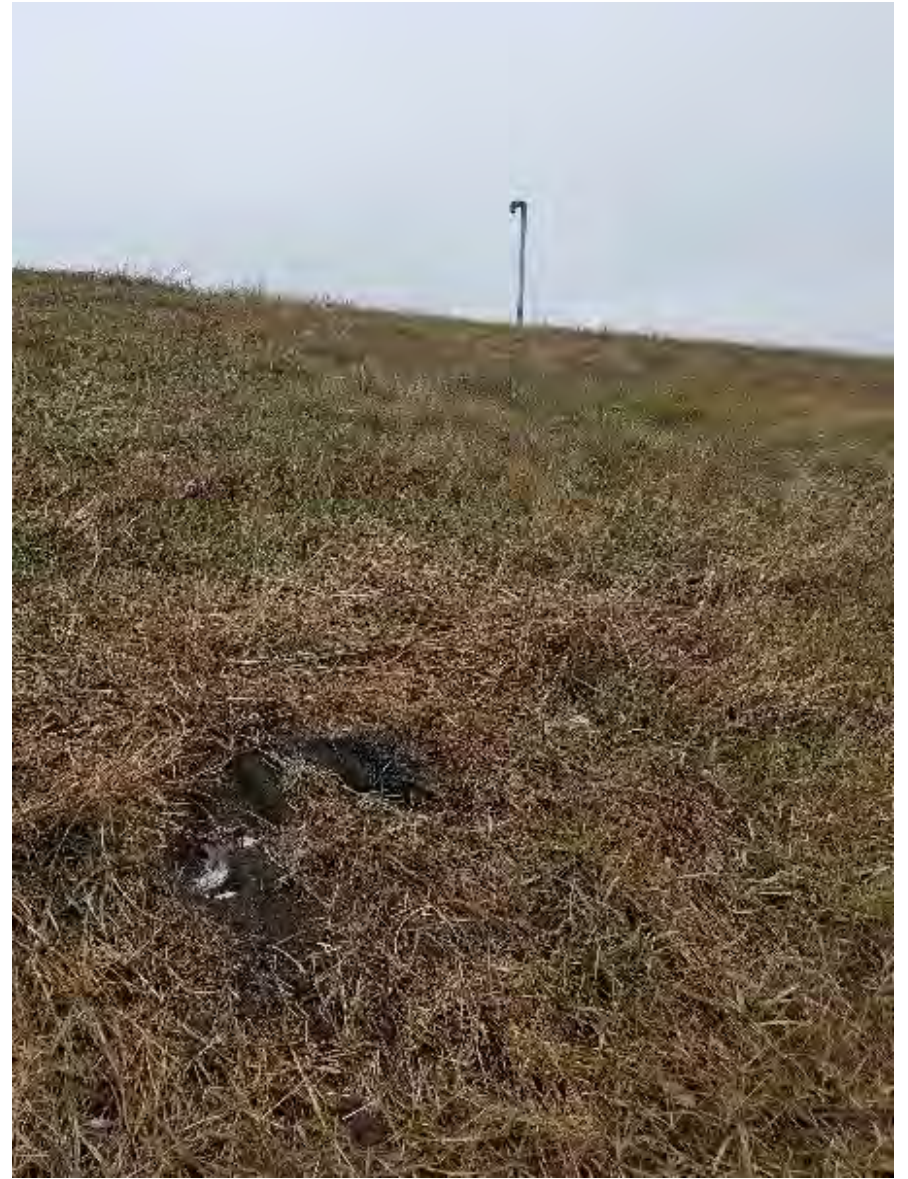
12. Hole and possible damage to liner, looking NW towards GV-8
