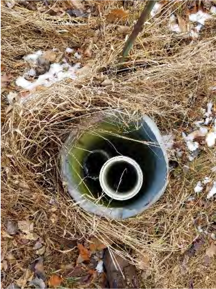
63. Unknown pipes in ground, not marked, N of B-96-17
