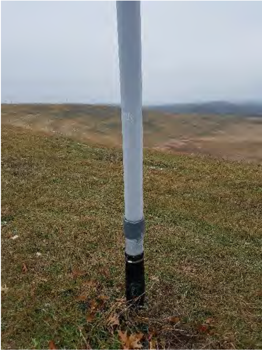
3. GV-3 boot needs repair, looking NW
