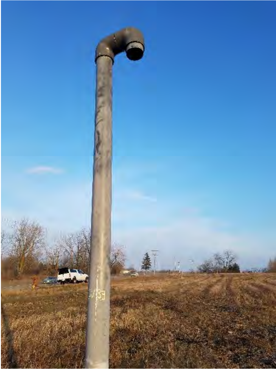
109. GV-33 missing vent screen, looking NE
