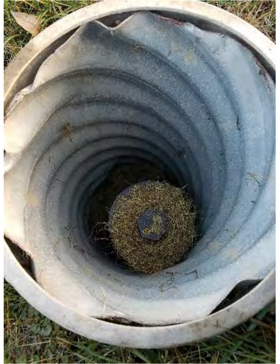
138. Inside unmarked northern LHW by leachate piping
