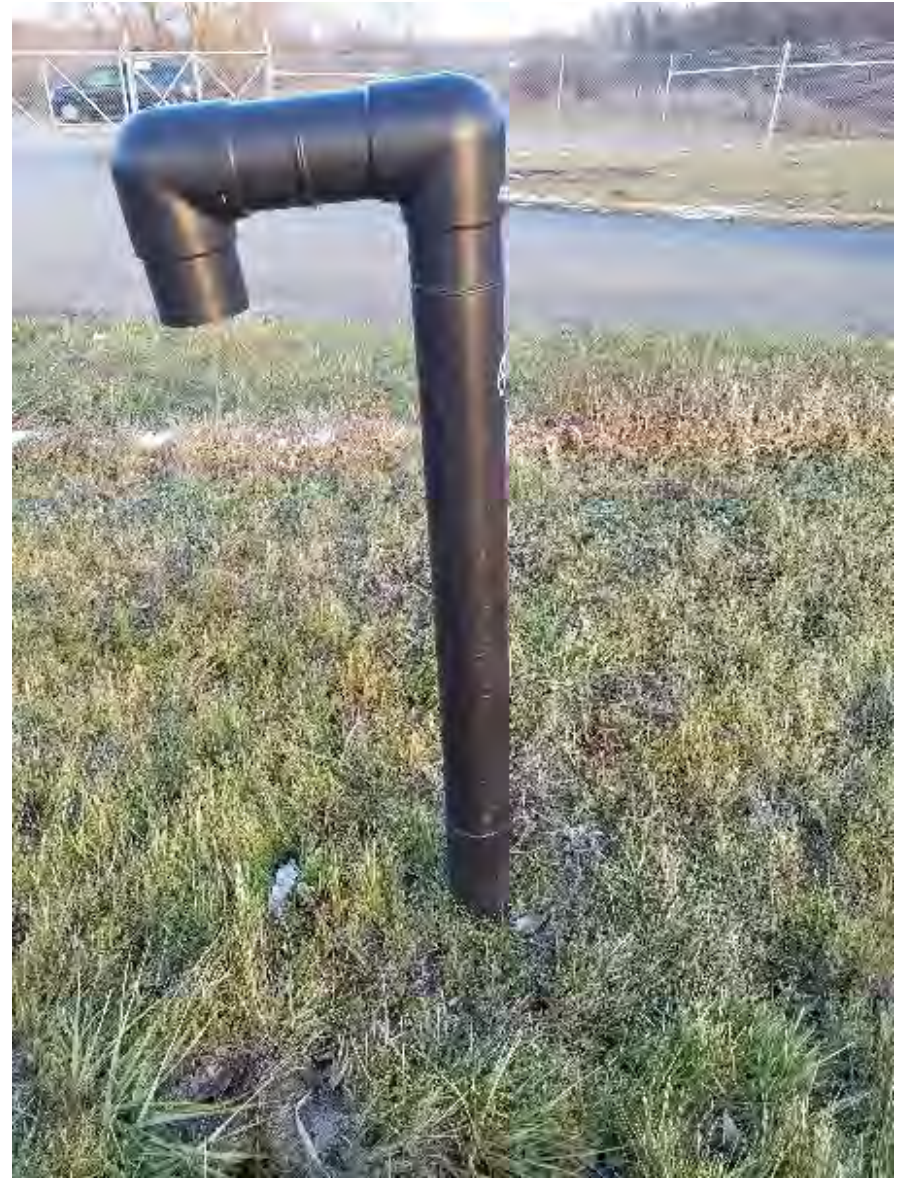
134. GV-1, no vent screen, looking E
