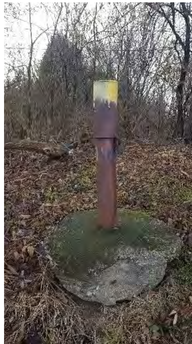
100. B-94-14A, looking W, erosion of soil around cement pad
