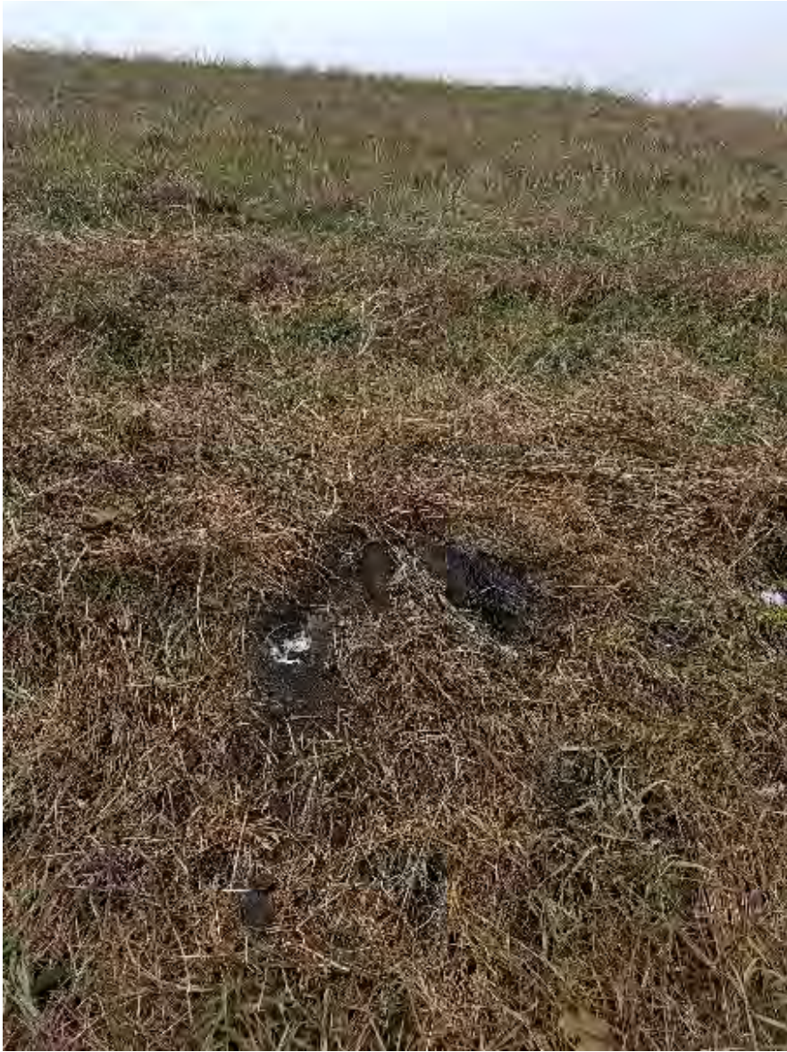
13. Hole and possible damage to liner SE of GV-8, looking W
