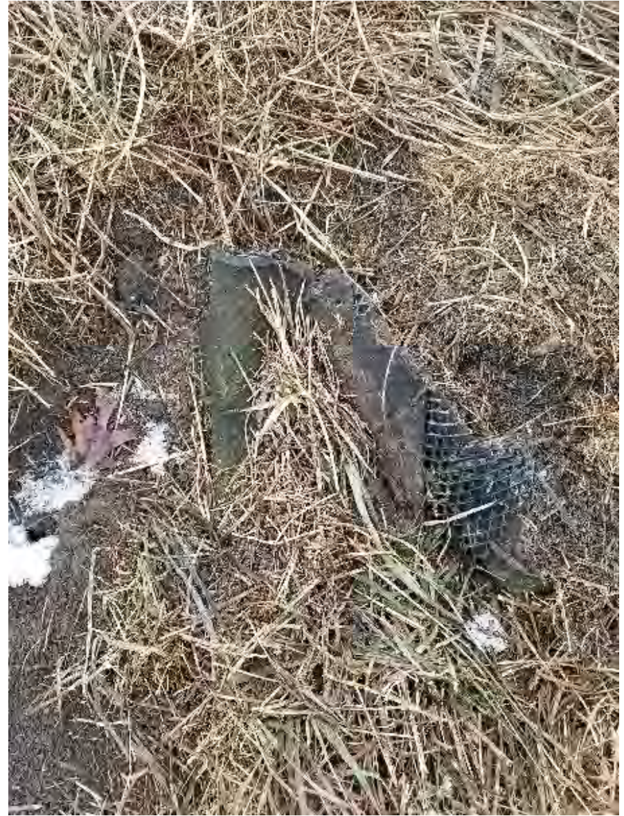
14. Hole and possible damage to liner
