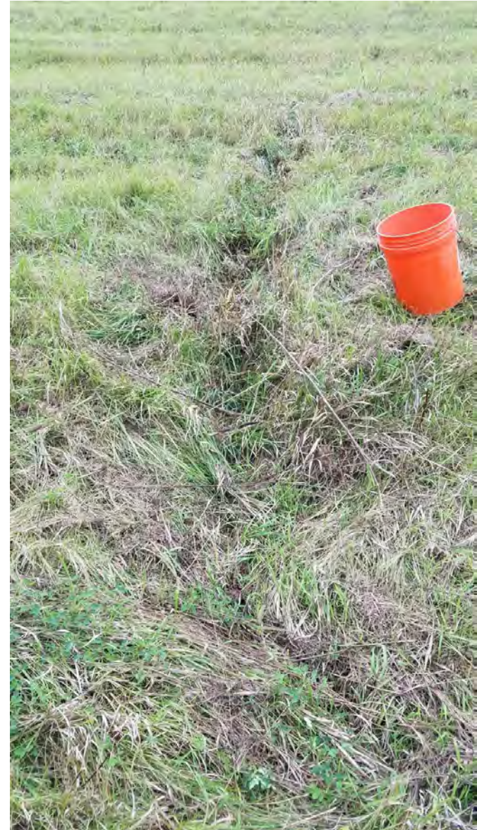
50. Erosion down hill face #7
