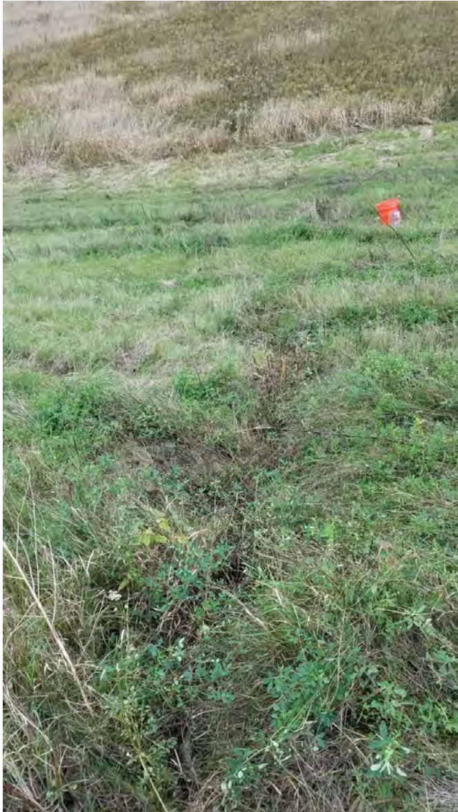
49. Erosion down hill face #6
