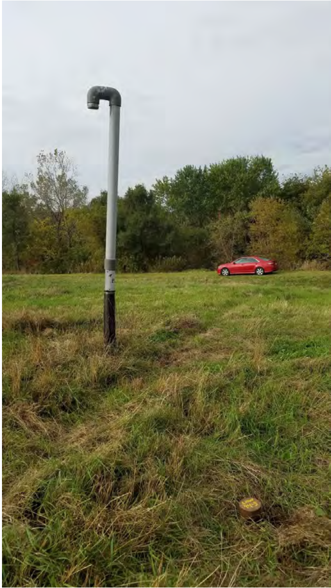
13. GV-4 Straight, LHW-94-3 unable to open
