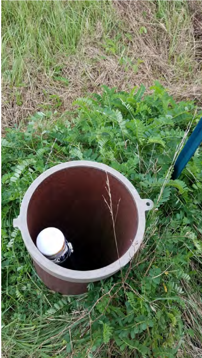
27. LHW-94-5 – no protective casing cover
