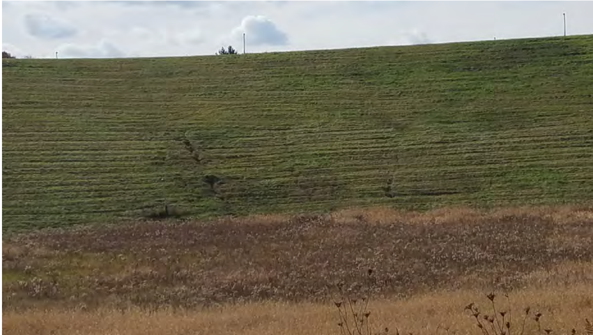
91. Extent of erosion down hillface
