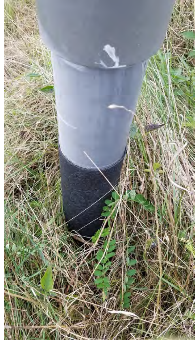
24. GV-129 Top of boot straight-no gaps, missing hose clamp
