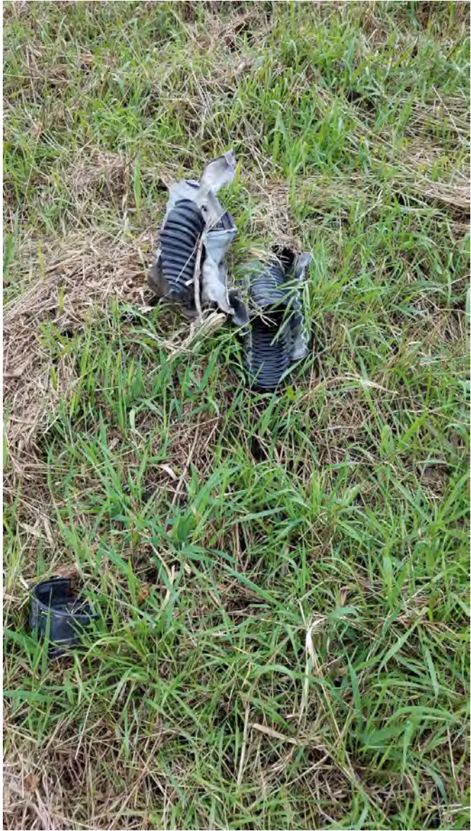
53. Damaged corrugated pipe
