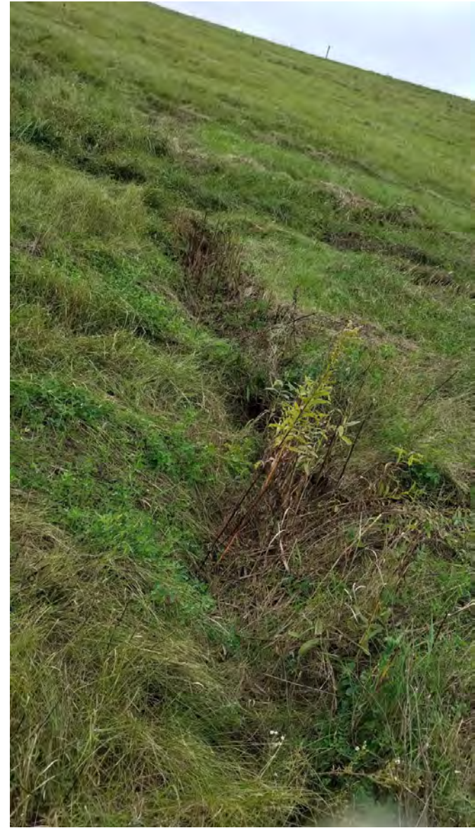
48. Erosion down hill face #5
