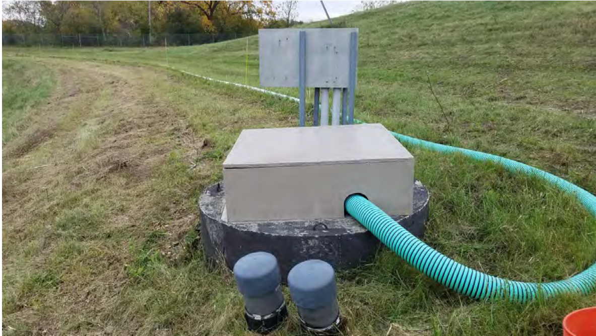
41. Leachate lift station #2
