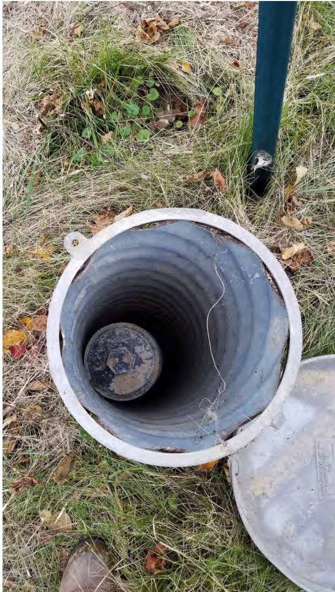
87. Inside unmarked vault – possible parts of old leachate system, near leachate piping
