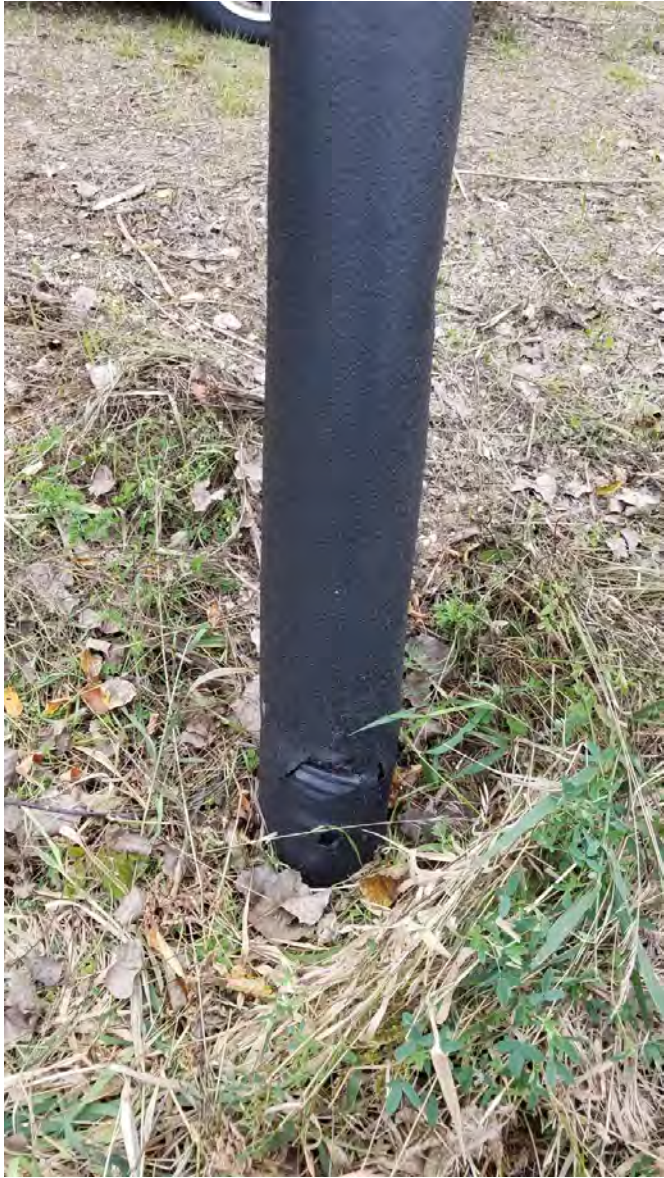
67. Tear in boot of unidentified LHW Southeast of GV-144 and North of GV-143
