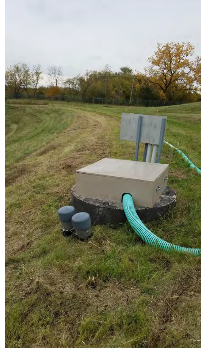
40. Leachate lift station
