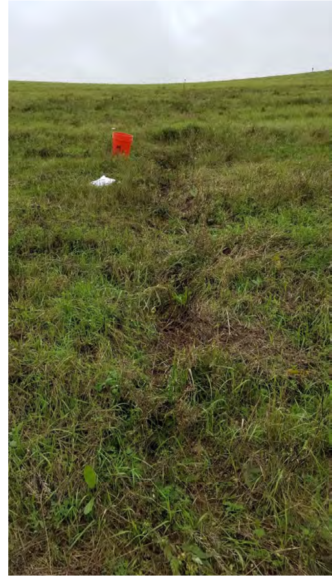
46. Erosion down hill face #3
