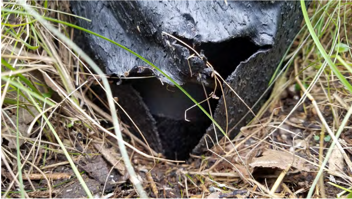
77. GV-137 tear at base
