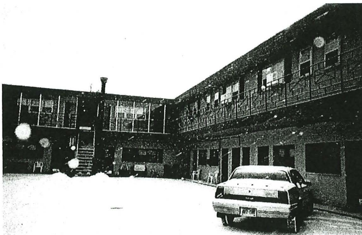
Photograph 3 – Additional view of interior courtyard and parking lot. Note chimney. This is one of the three asbestos chimney pipes that are found on the premises.
