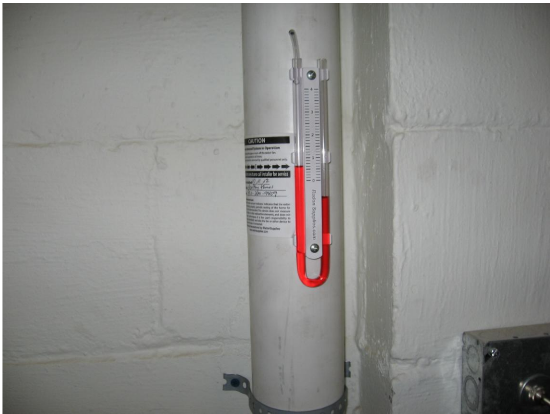
Photograph #: 6 Date: 10/11/2012 Direction: System #1 Subject: U-tube monometer above eastern suction point
