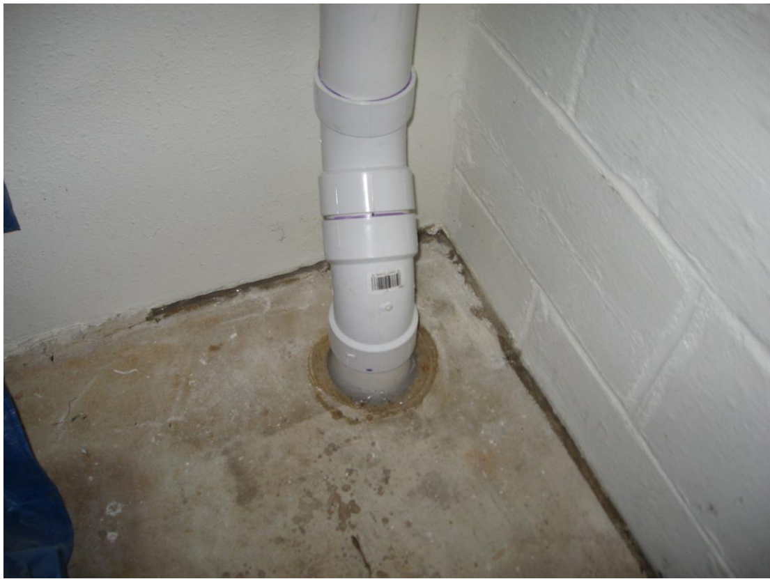
Photograph #: 7 Date: 10/11/2012 Direction: System #2 Subject: Sub-slab depressurization system suction point
