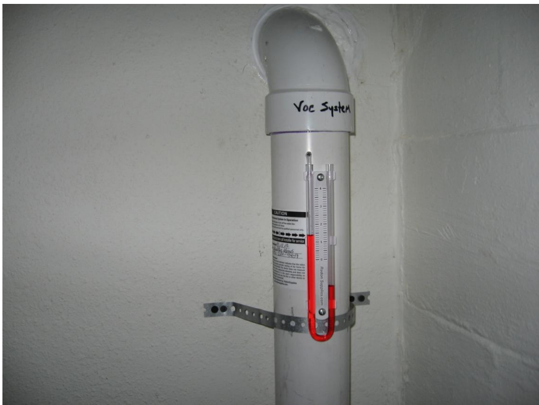
Photograph #: 8 Date: 10/11/2012 Direction: System #2 Subject: U-tube monometer
