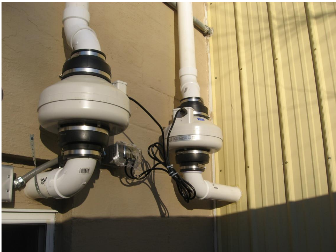
Photograph #: 10 Date: 10/11/2012 Direction: Facing east Subject: Fans mounted on west side of building
