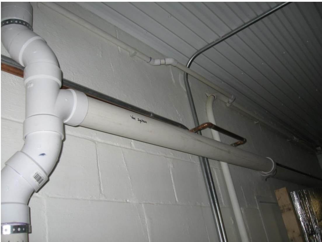
Photograph #: 4 Date: 10/11/2012 Direction: System #1 Subject: Piping manifolded together
