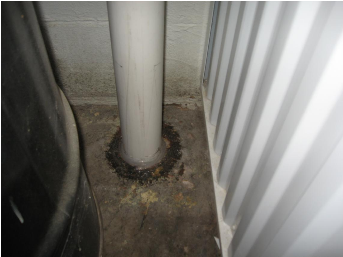
Photograph #: 3 Date: 10/11/2012 Direction: System #1 Subject: Sub-slab depressurization system western suction point
