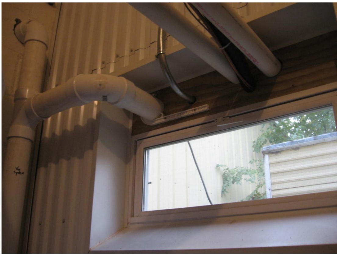
Photograph #: 5 Date: 10/11/2012 Direction: System #1 Subject: Piping routed to exterior where fan is mounted
