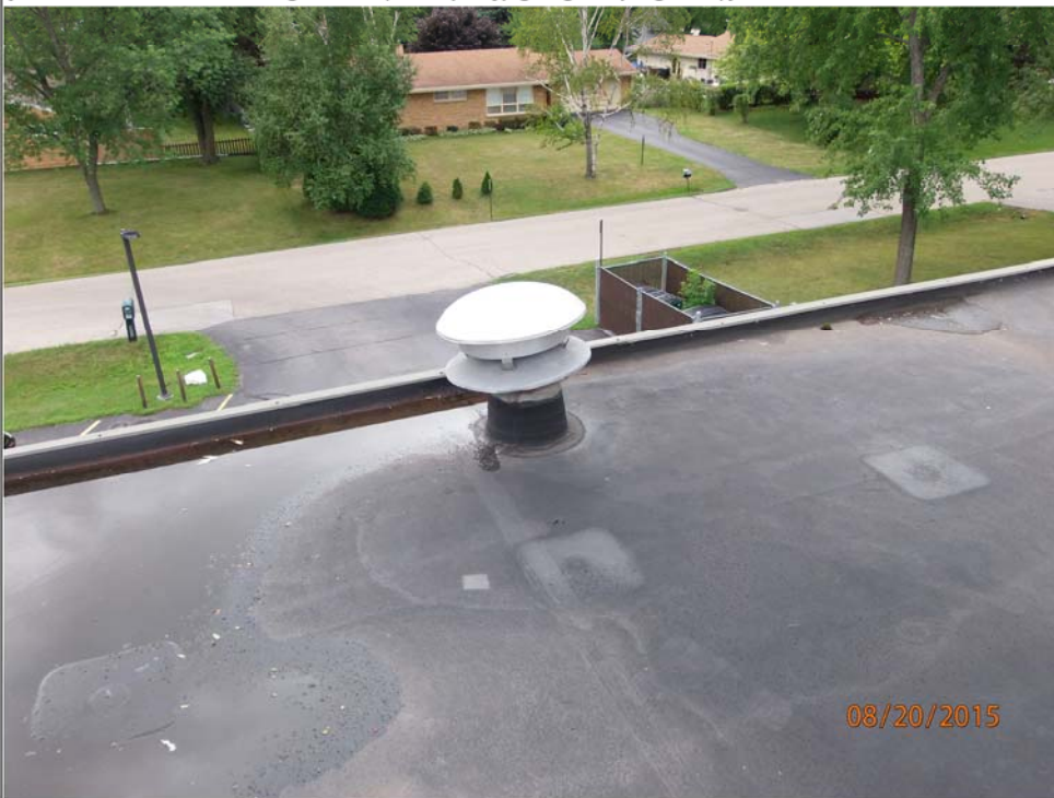
Title: Positive air exchanger vent stack on roof.
