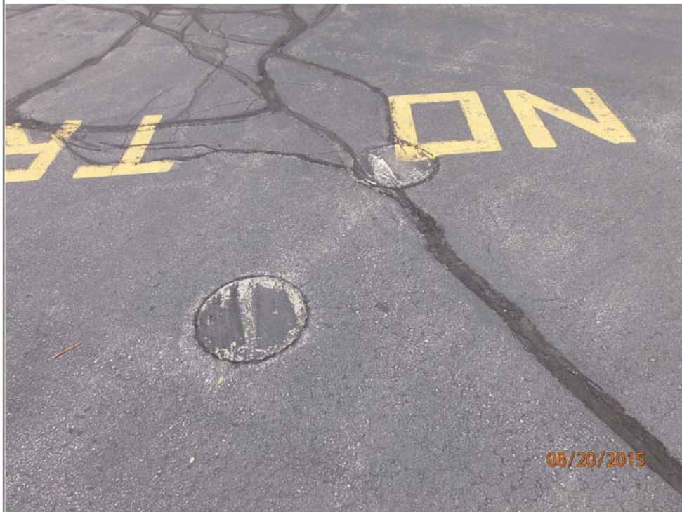
Title: Abandoned wells in parking lot.
