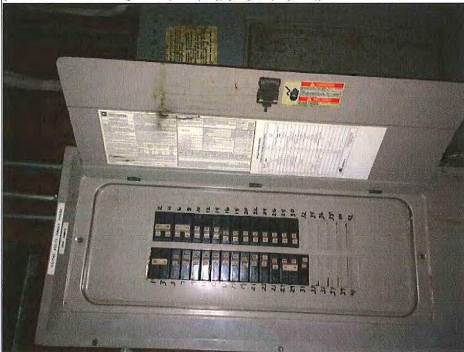
Title: Circuit breaker box - vapor mitigation system breaker location labeled
