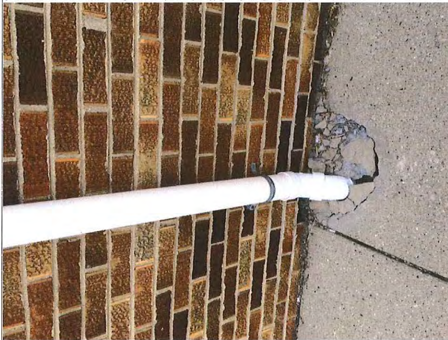
Title: Vent pipe exit from building - repair needed.
