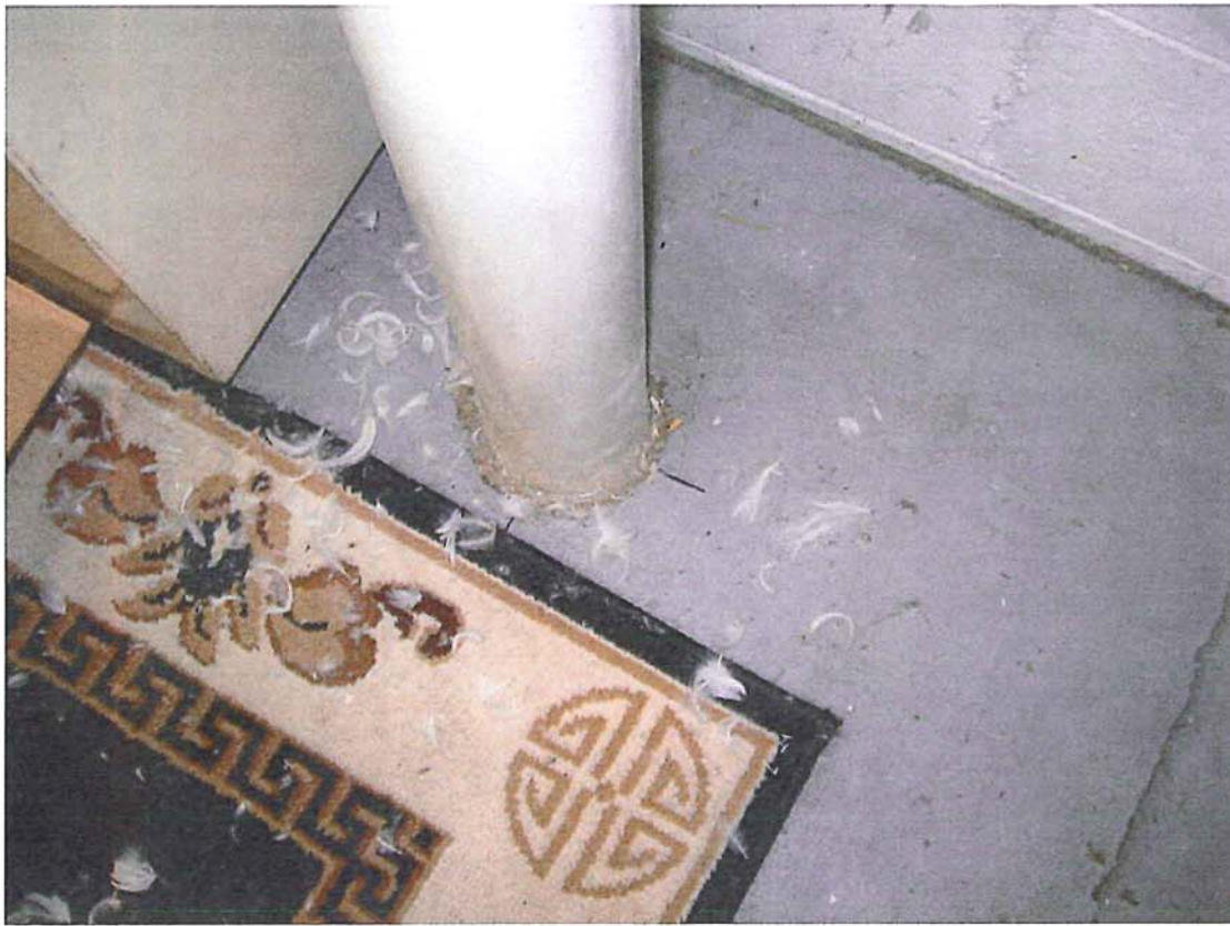
Photograph #: 1 Date: 5/24/2011 Direction: Inside site building Subject: Sub-slab depressurization system suction location
