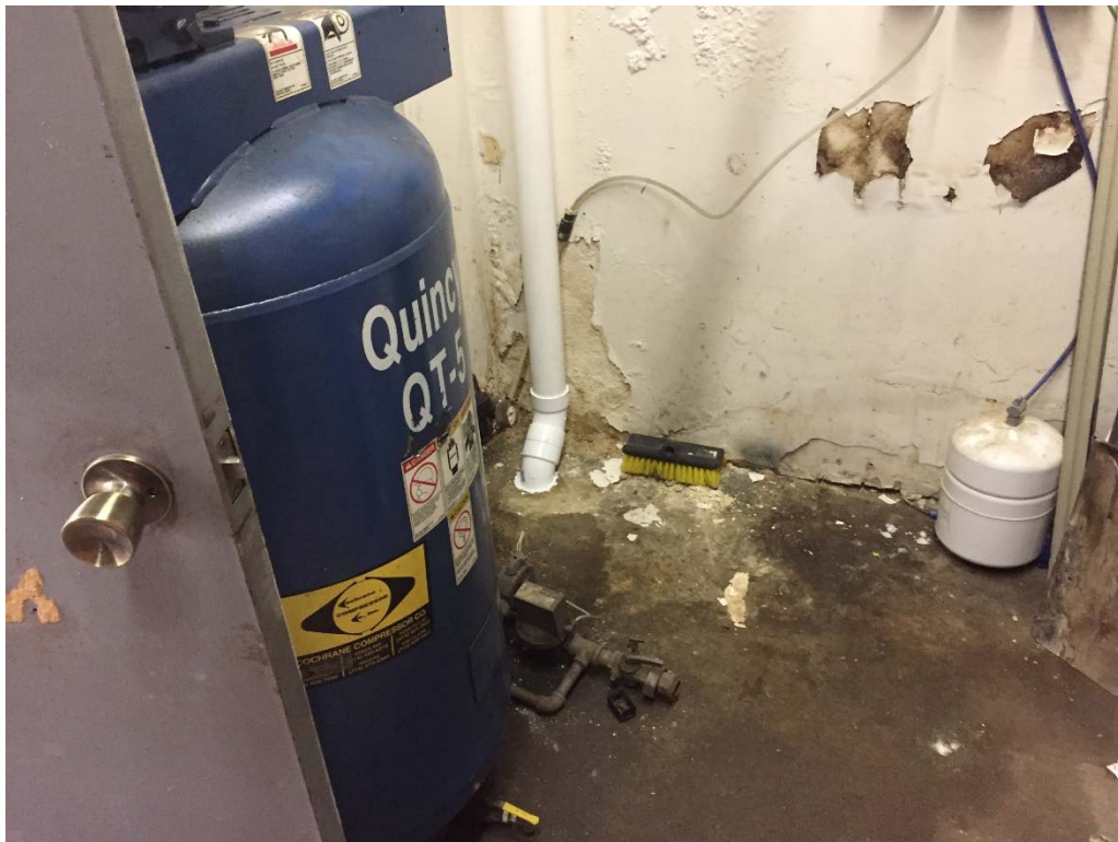
Suction Point EP-4 in boiler room
