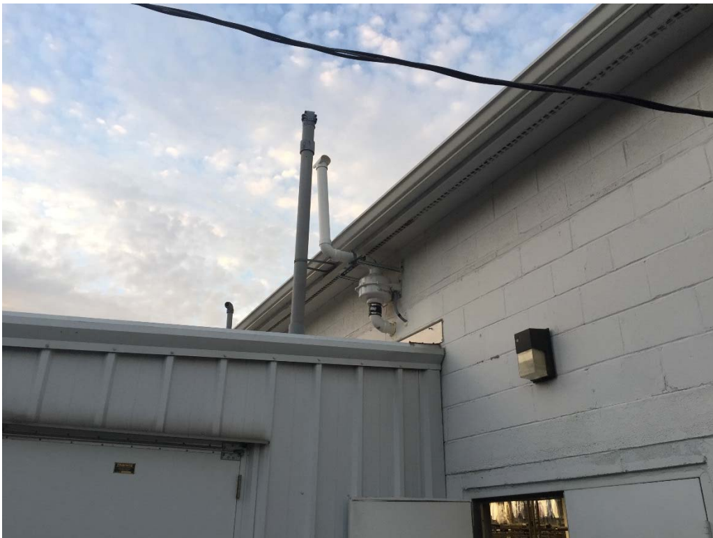
Fan on south wall of building
