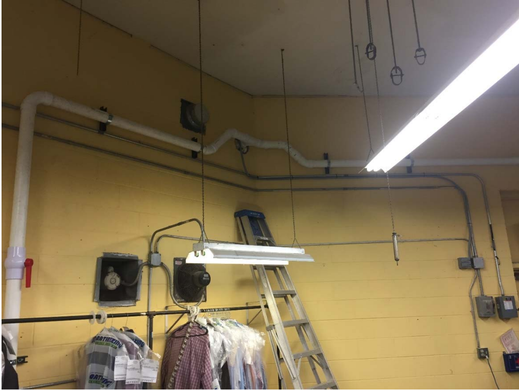
Mitigation system piping
