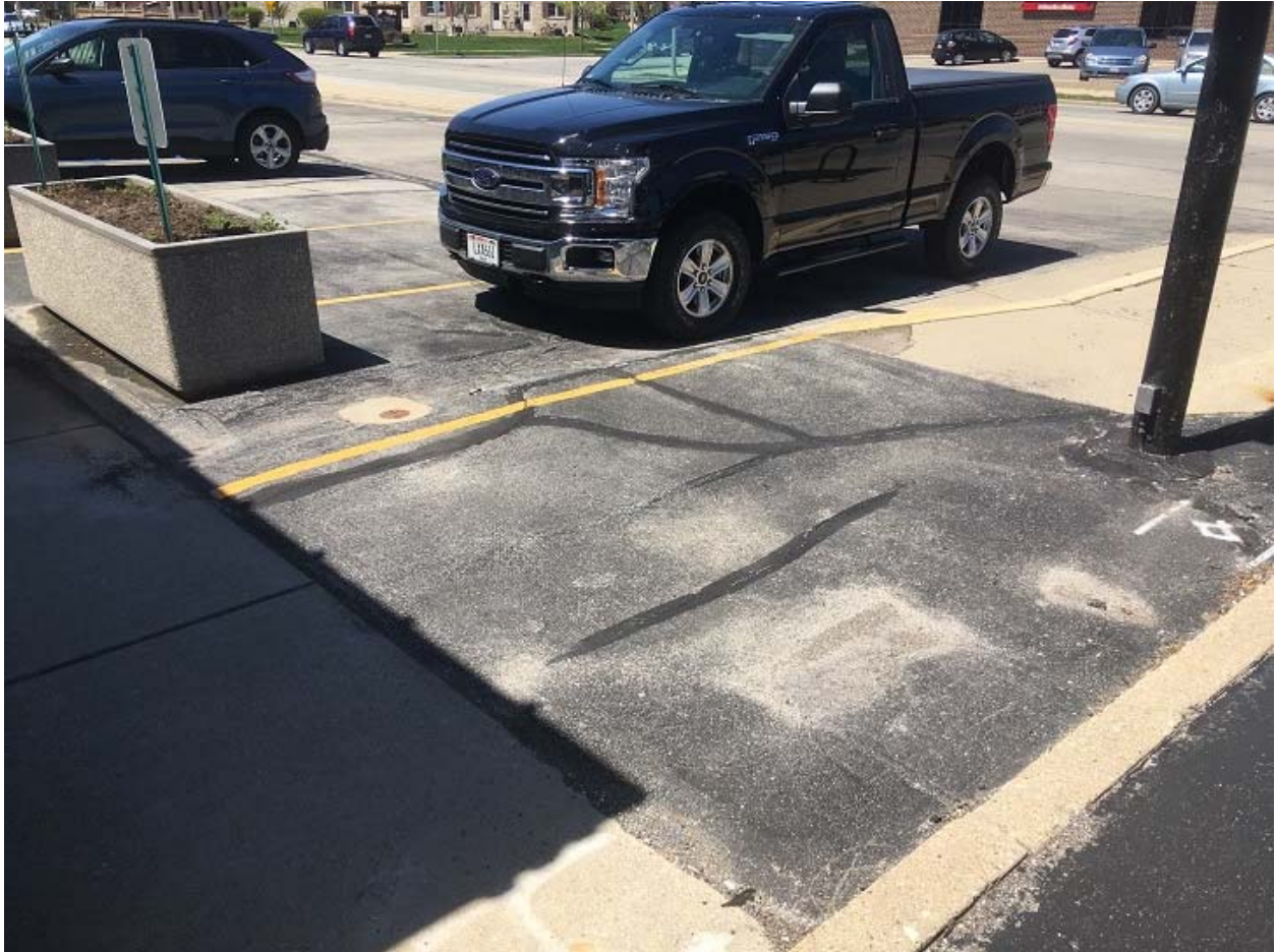
View of asphalt/concrete located in the north parking area. View is to the northwest.
