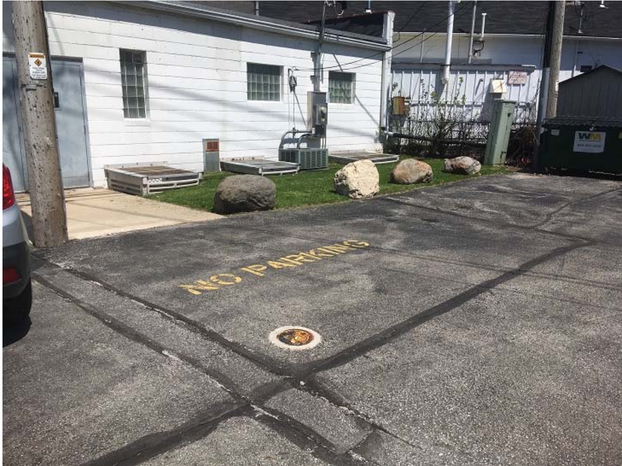
View of the asphalt/concrete, building foundation, and vegetated areas on the south side of the Property building. View is to the northeast.
