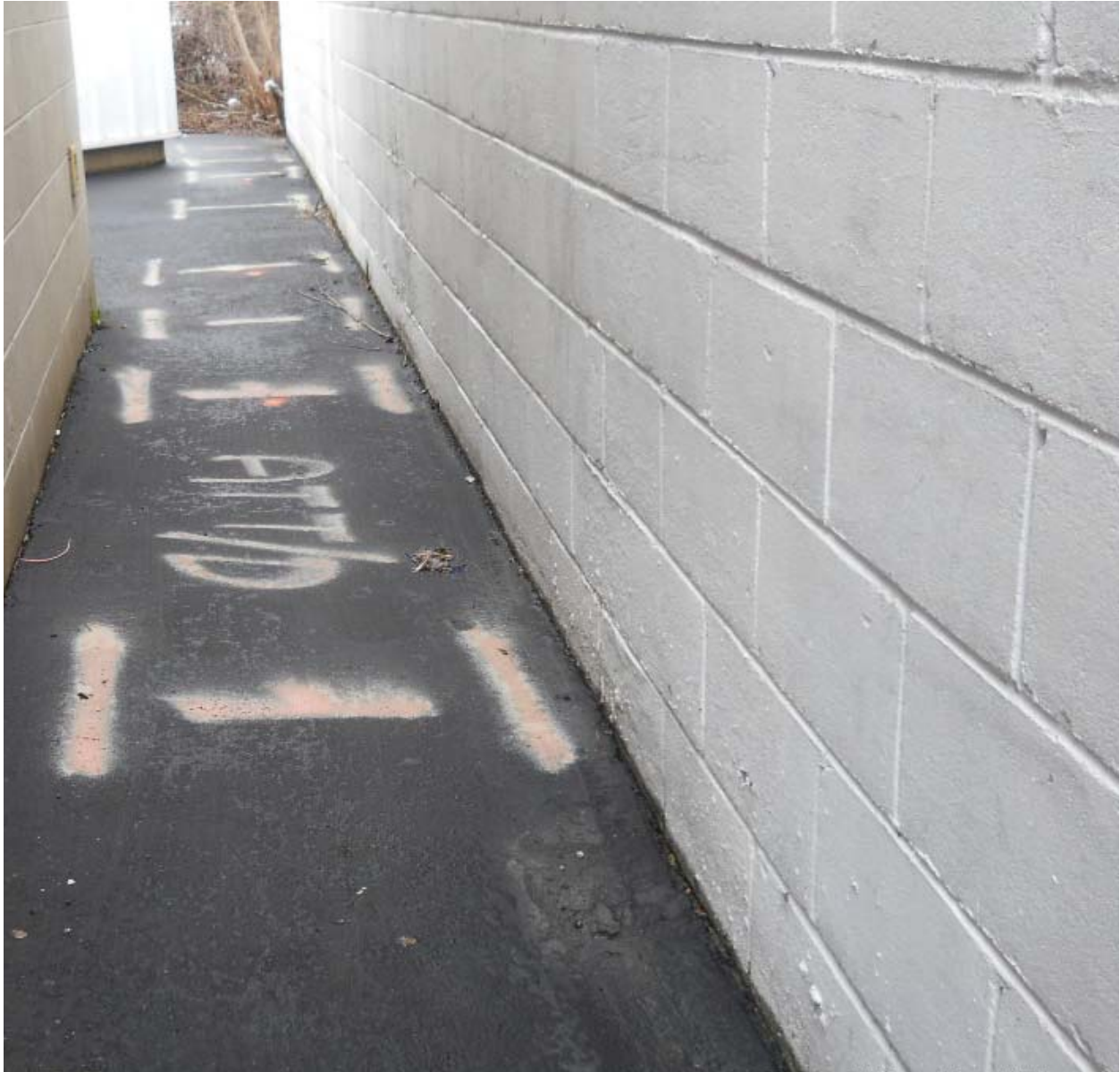
View of the east Property building foundation. View is to the south.
