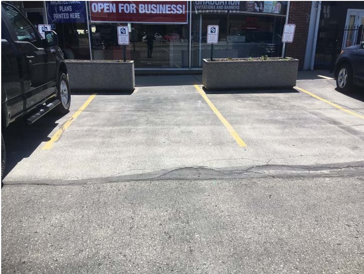
View of the asphalt/concrete in the north parking area and building foundation. View is to the south.
