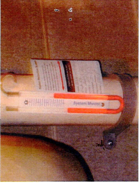
Vacuum Measuring Sight Tube Showing Reading while Mitigation System is Operating Properly
