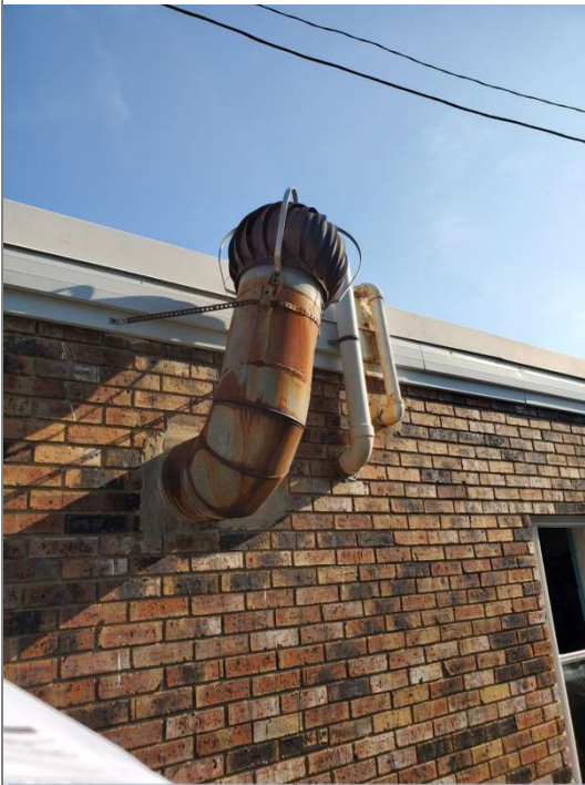
Title: VMS Exhaust Stack, (White PVC) Rear of Building
