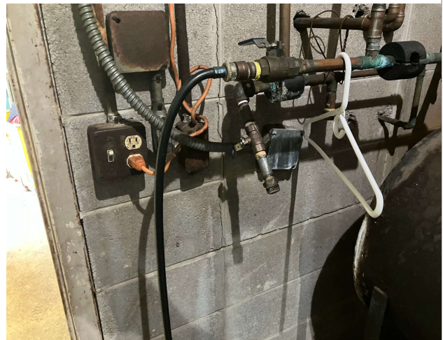
Description: Power cord
