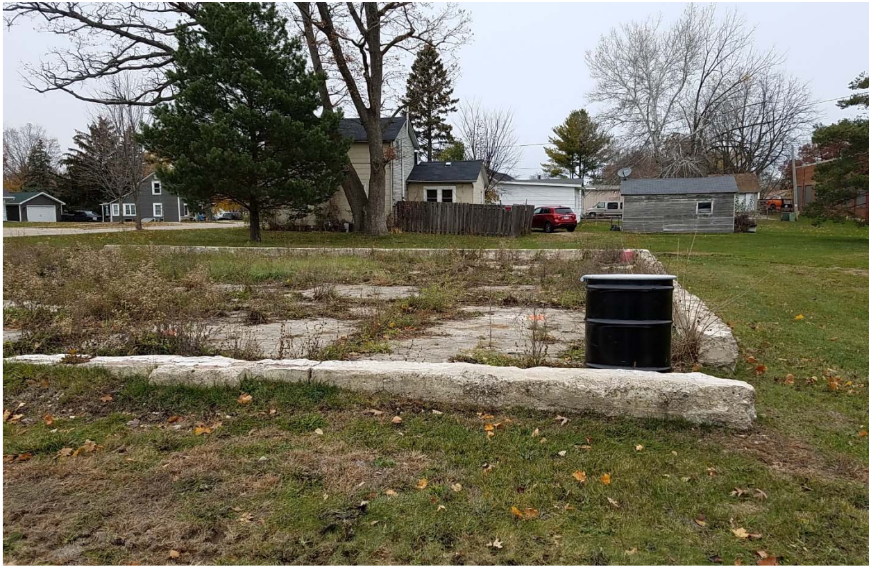
Overview of planned excavation area, facing north. Concrete features are the foundation walls and slab of the former building.
