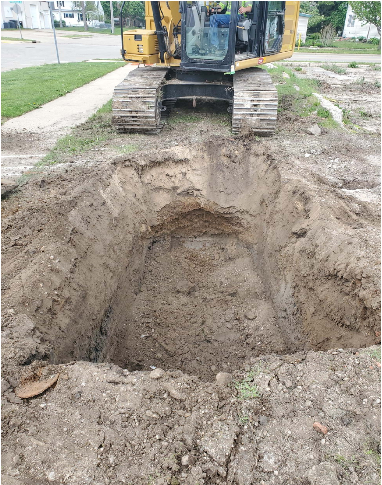
Overview of the separate excavation area between the former building and 1 st Street right-of-way, facing west.
