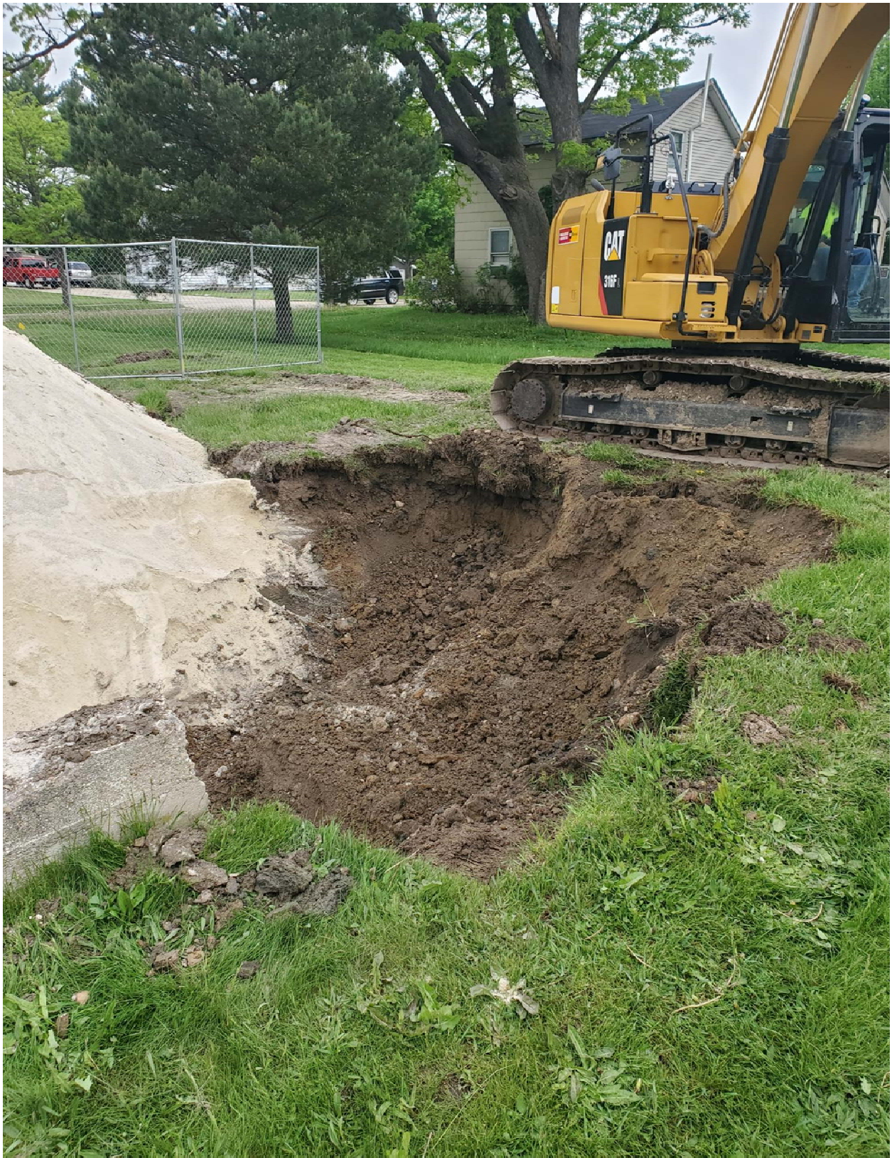
Northeast corner of the excavation expanded beyond the foundation to remove highly contaminated soil, facing northwest.
