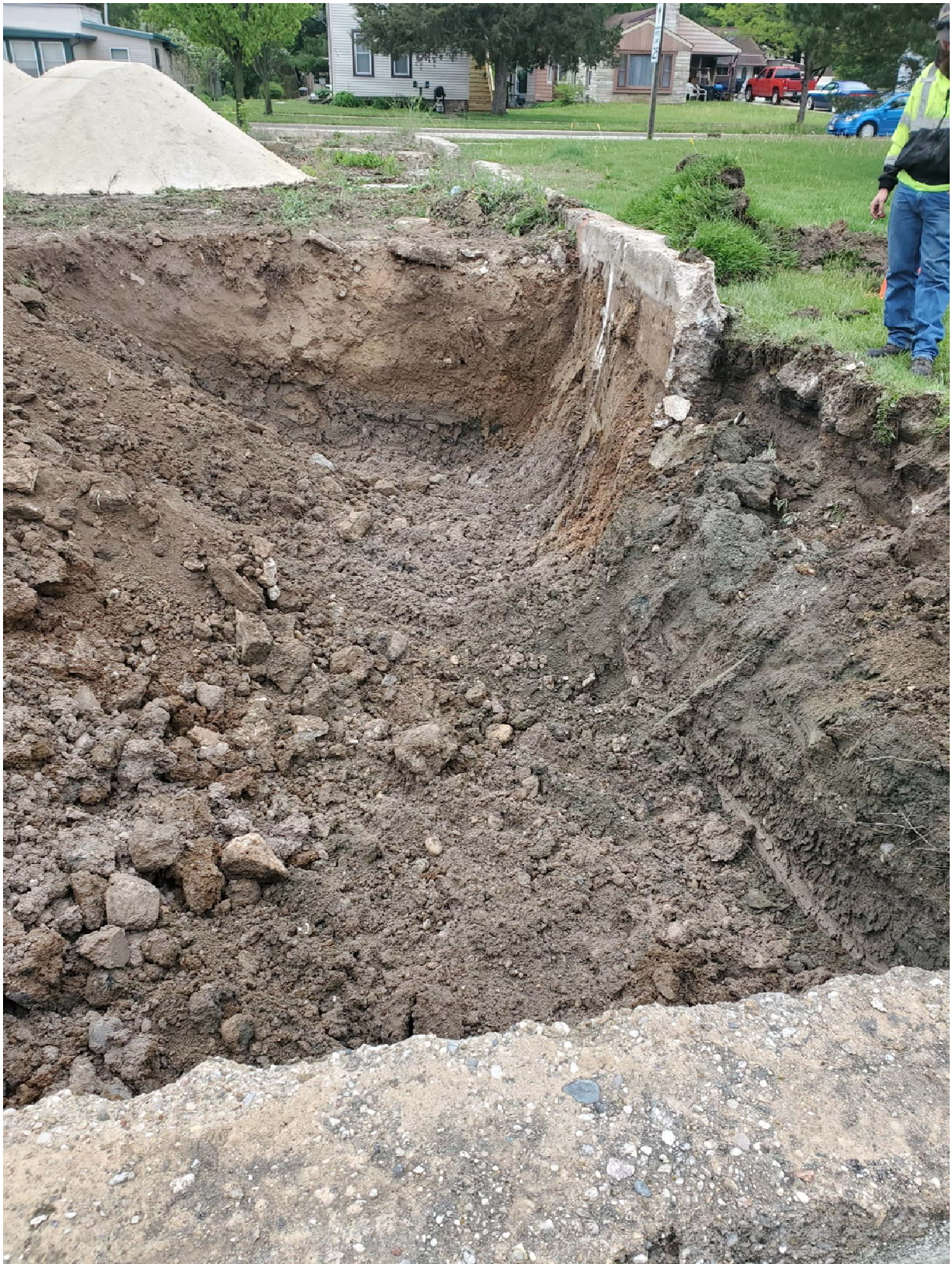
North end of the excavation, facing west. Sections of the footing in this area were removed to allow excavation of highly contaminated soil beneath.
