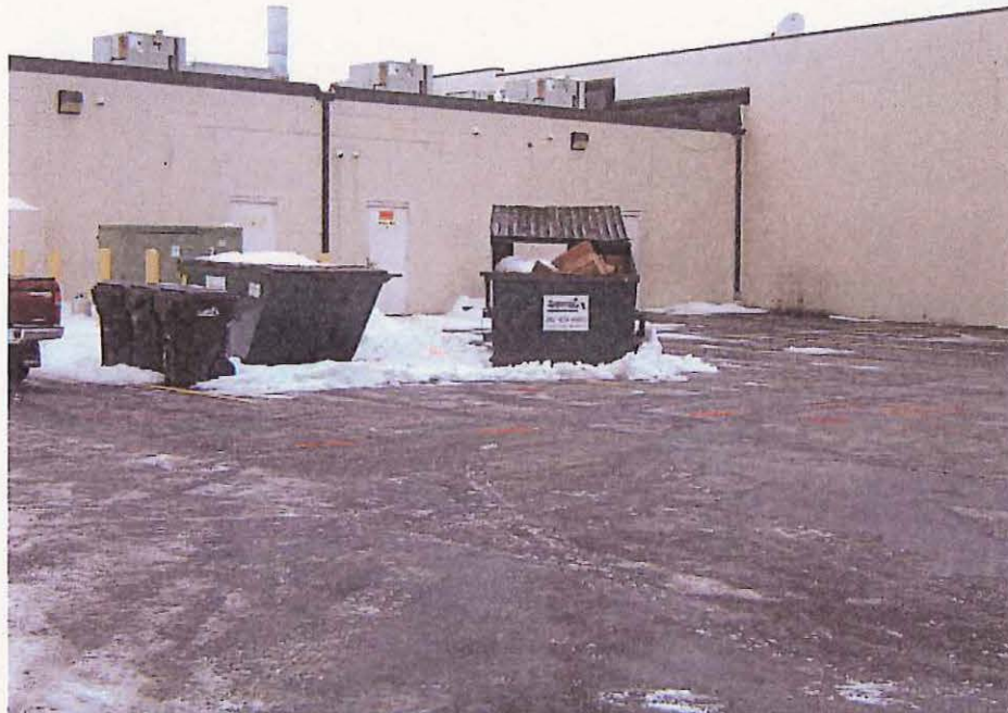
Photo No. 5: Photo showing asphalt pavement behind the dry cleaners tenant space, view to the northwest; photo taken on December 13, 2005.
