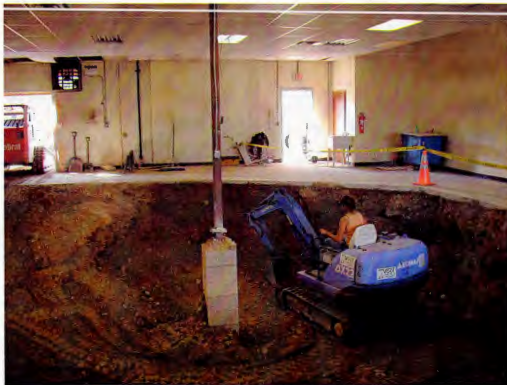
Photo 2: Soil was excavated using a mini-excavator and bobcat. View to the south (back).
