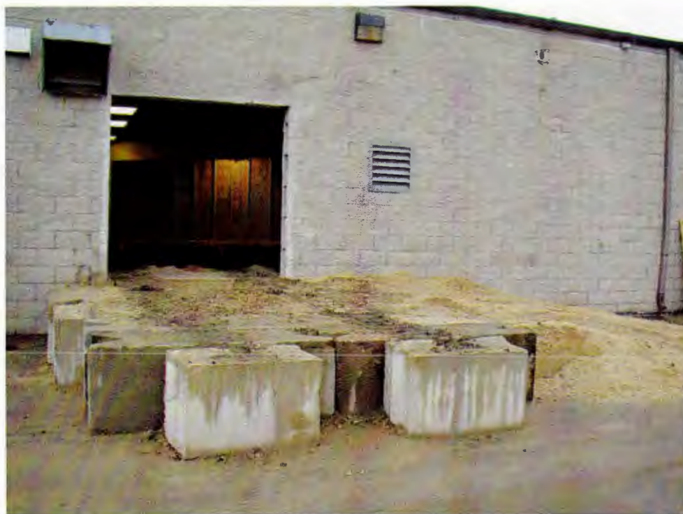
Photo 3: A hole was cut in the back of the building, and concrete blocks used to make an elevated platform, so the soil could be located by the bobcat into trucks.
