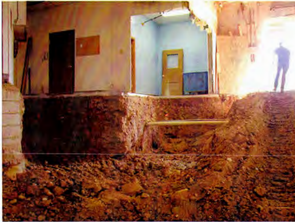
Photo 5: Excavation was conducted around the sanitary sewer and water lines in many locations. The orange flag in the background, behind the utility lines, marks a soil sample location. View to the southeast.
