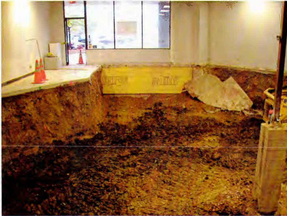
Photo 7: In some cases excavation extended all the way to the concrete block foundation, exposing insulation. View to the north (front of building).
