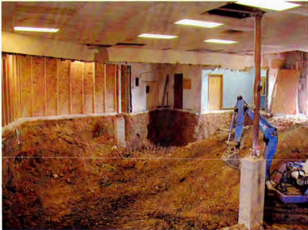
Photo 1: Walls between the tenant suites were removed (in this case between Suites 8 and 10) as necessary to access contaminated soil for excavation purposes. View to the east southeast.
