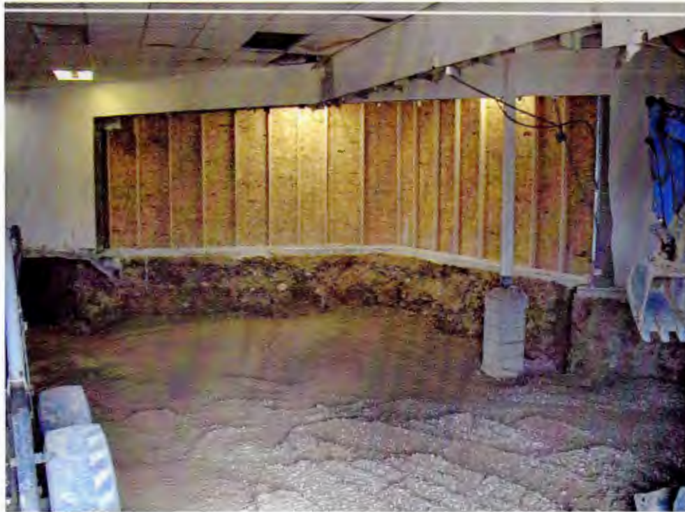
Photo 8: The excavation was backfilled with limestone screenings in lifts, and compacted. View to northeast.
