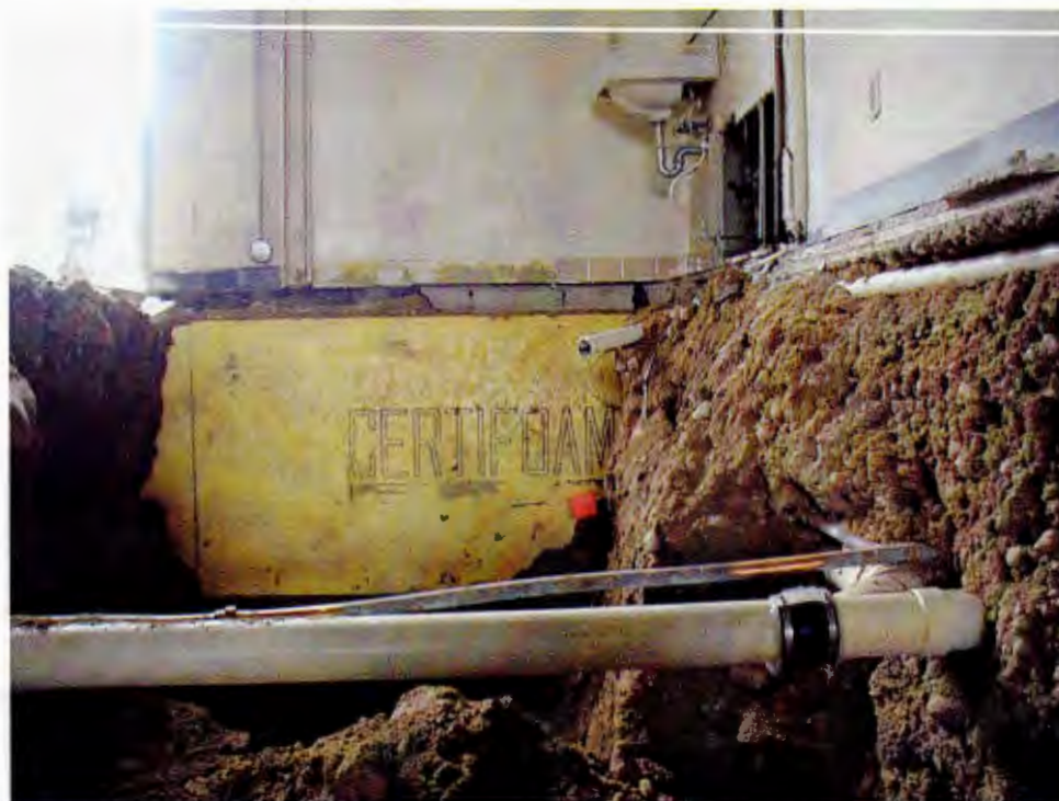
Photo 4: It was necessary to excavate around utility lines with a shovel. The water and sanitary sewer piping from the bathroom (SW corner) connects to the main water and sewer lines.
