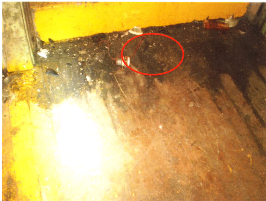
Photograph No.: 12 Photographer: Caitlin Ruza Area: Bldg I-Transformer TDD Number: TO-05-10-12-0002 Contract: EP-S5-10-10, OTIE Date: January 24, 2011 Site Name & Location: Mirro-Spirtas Site, Manitowoc, Manitowoc County, Wisconsin Photograph Subject: MS-WP-7 collected from stained area outside of entranceway to the transformer room in Building I (approximate sample area shown)
