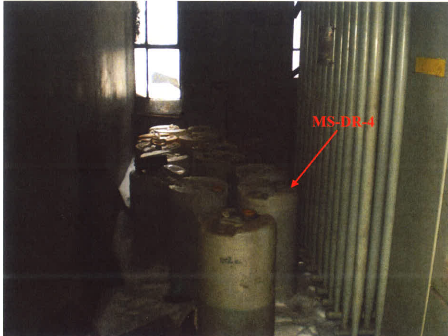
Photograph No.: 17 Photographer: Caitlin Ruza Area: Building K-Transformer TDD Number: TO-05-10-12-0002 Contract: EP-S5-10-10, OTIE Date: January 24, 2011 Site Name & Location: Mirro-Spirtas Site, Manitowoc, Manitowoc County, Wisconsin Photograph Subject: MS-DR-4 was collected from the second drum back from the front of the photo on the right. These 14 drums are located inside the transformer room in Building K
