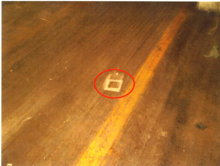
Photograph No.: 10 Photographer: Caitlin Ruza Area: Bldg I-Transformer TDD Number: TO-05-10-12-0002 Contract: EP-S5-10-10, OTIE Date: January 24, 2011 Site Name & Location: Mirro-Spirtas Site, Manitowoc, Manitowoc County, Wisconsin Photograph Subject: MS-WP-5 collected from outside of saturation staining on flooring outside of the transformer room in Building I (template area shown)
