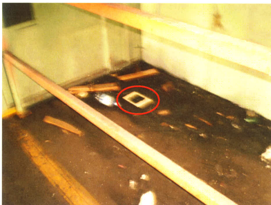
Photograph No.: 8 Photographer: Caitlin Ruza Area: Building I-Transformer TDD Number: TO-05-10-12-0002 Contract: EP-S5-10-10, OTIE Date: January 24, 2011 Site Name & Location: Mirro-Spirtas Site, Manitowoc, Manitowoc County, Wisconsin Photograph Subject: MS-WP-3 collected from stained area of small railed in section adjacent to the transformer room in Building I (template area shown)
