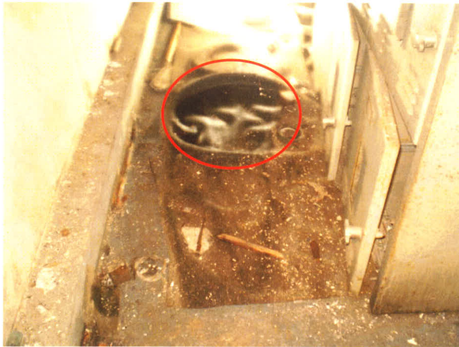
Photograph No.: 11 Photographer: Caitlin Ruza Area: Bldg I-Transformer TDD Number: TO-05-10-12-0002 Contract: EP-S5-10-10, OTIE Date: January 24, 2011 Site Name & Location: Mirro-Spirtas Site, Manitowoc, Manitowoc County, Wisconsin Photograph Subject: MS-WP-6 collected from puddle on plastic matting in the transformer room in Building I (approximate sample area shown)
