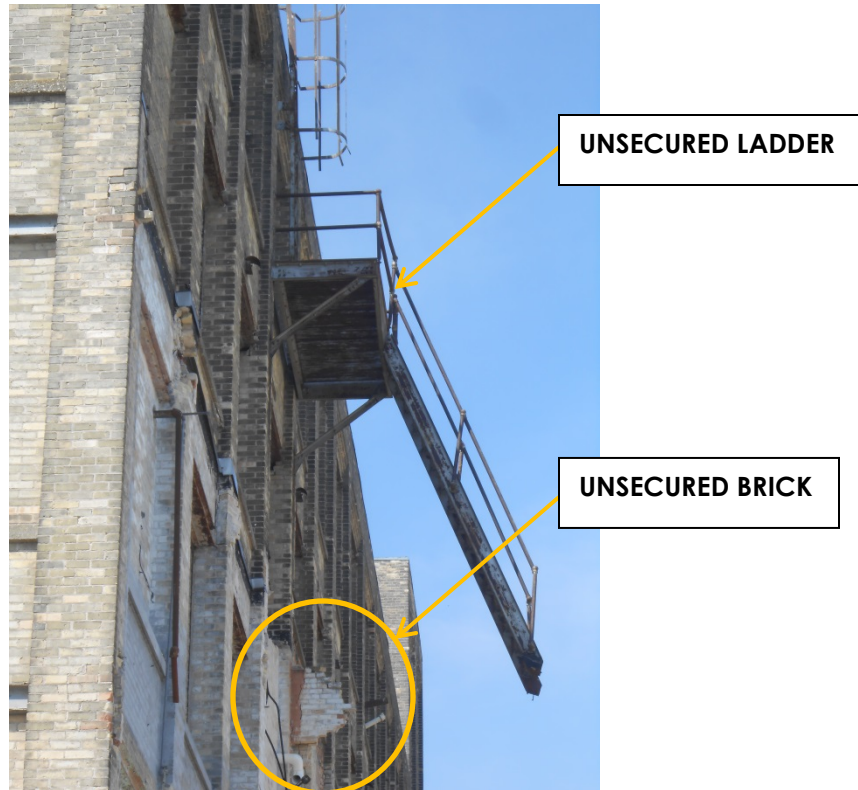
Photo No. 2 – Overhead Hazards
