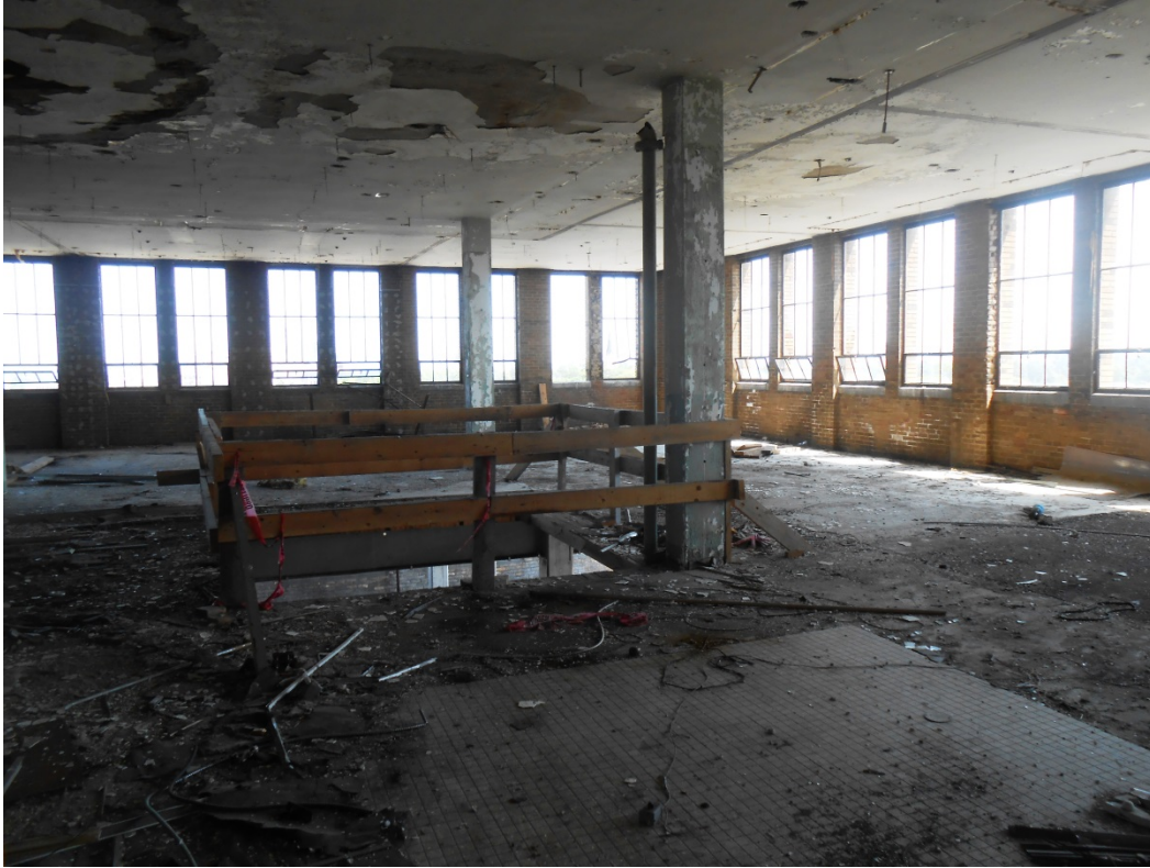
Photo No. 3 – Existing Demolition Debris Opening
