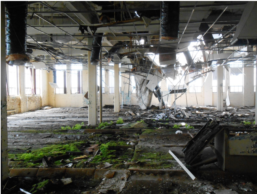
Photo No. 4 – Collapsed Roof in Southwest Corner
