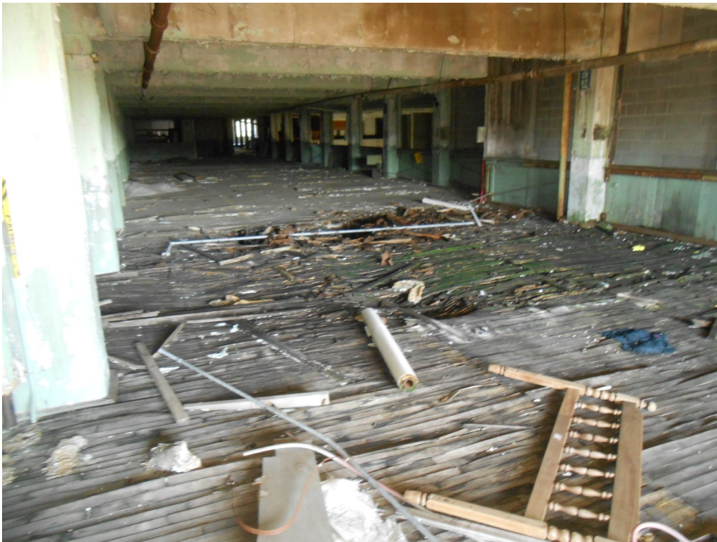
Photo No. 6 – Unsafe Floor Area on 2 nd Floor
